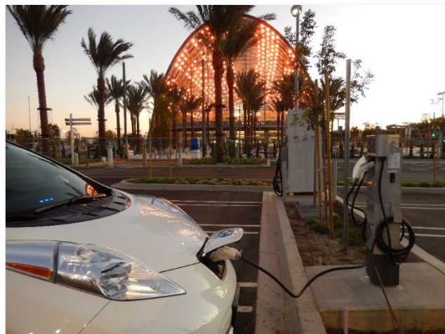
Photo 7: Charging Stations at Anaheim Regional Transportation Intermodal Center
