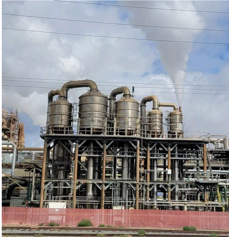
Process heating system at Woodland's tomato processing facility. Source: Pacific Coast Producers
