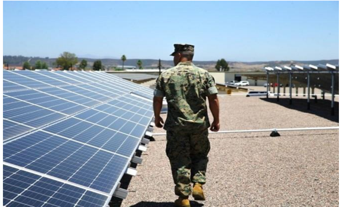
A United States Marine walks by solar panels at MCAS Miramar Source: US Marine Corps
