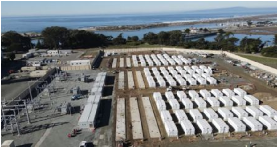
Figure 1 | Elkhorn Battery at Moss Landing (Source: Tesla)
