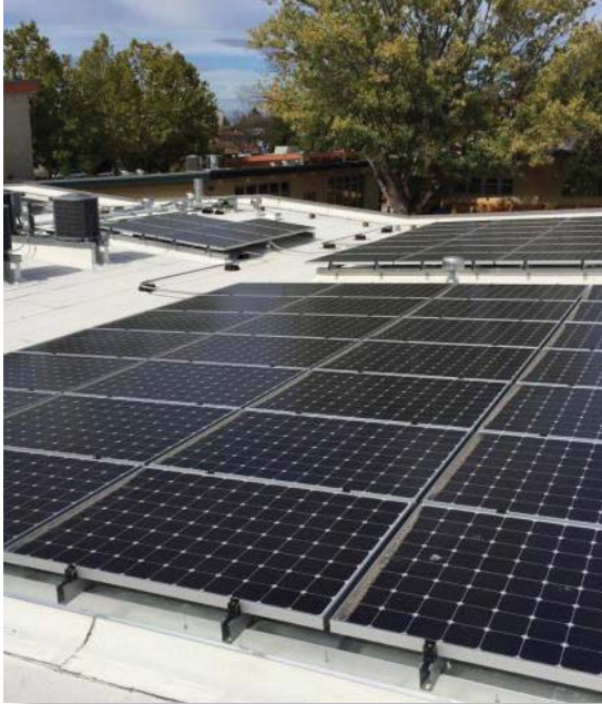
Solar Roof at Castlemont School
