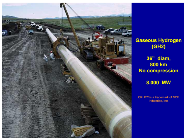
Figure 18. [62] CRLP test section, TransCanada, Alberta, ~ 2002. Weld joints on X70 are field overwrapped with FRP and cured before overpressure hydrotesting, which deforms steel core pipe. Thus, at MAOP steel is still in compression, and may be less susceptible to HE, HCC. Not tested for GH2 in VER service.
