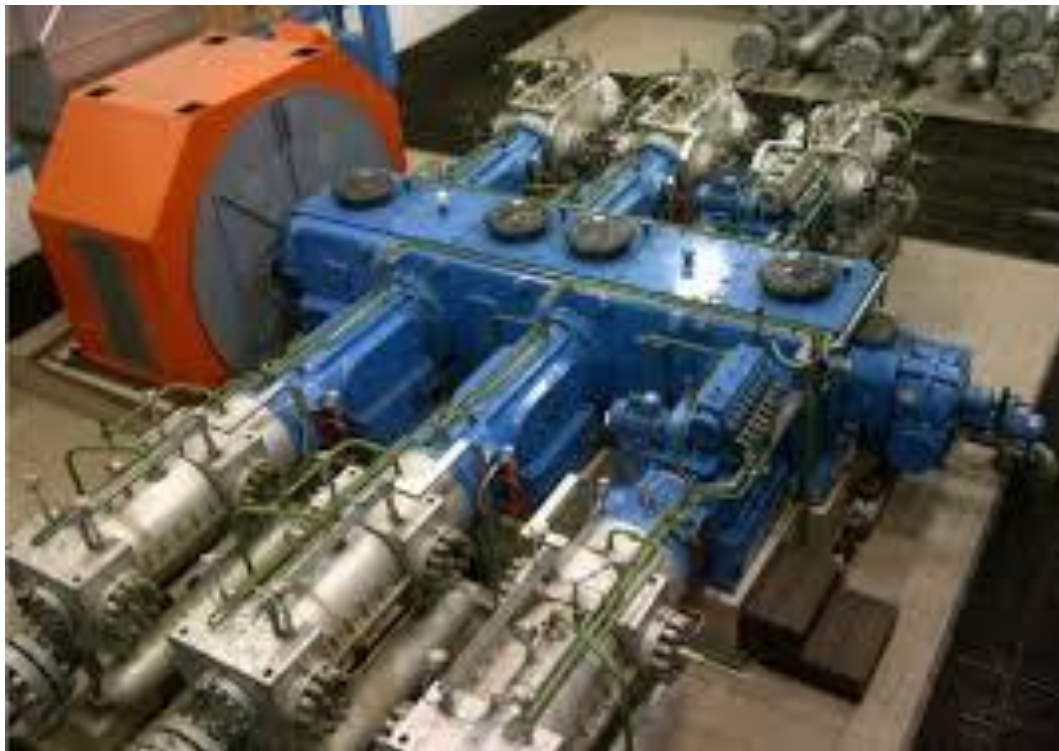
Figure 27. Typical reciprocating, positive-displacement, un-lubricated, GH2 compressor; electric motor drive.
