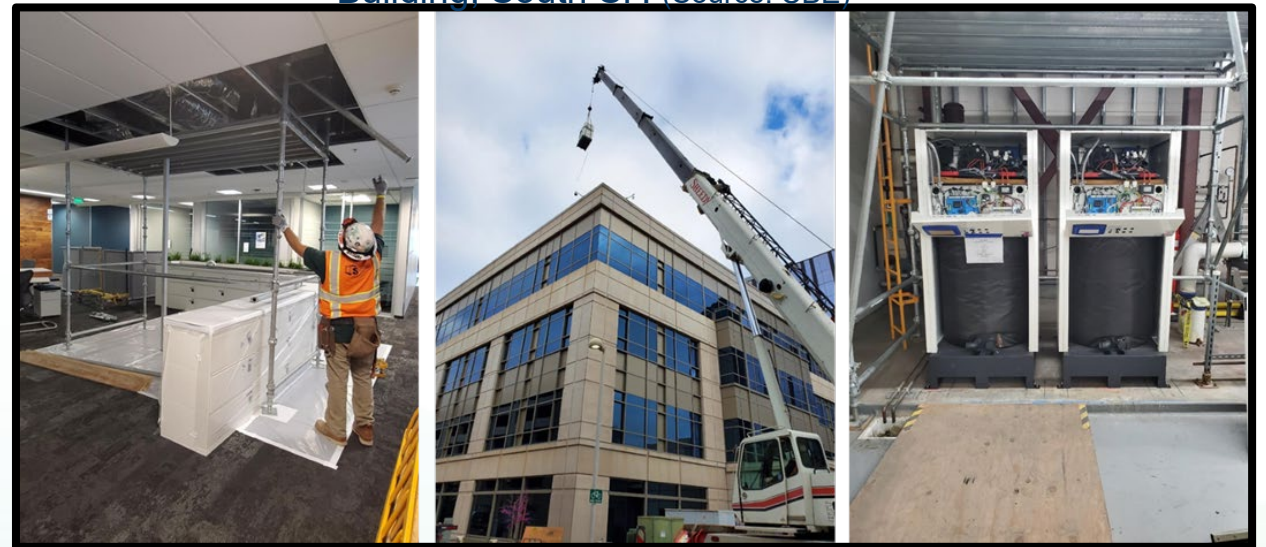
Boiler and Variable-Air-Volume Retrofits at the Genentech Building, South SF. (Source: CBE)
