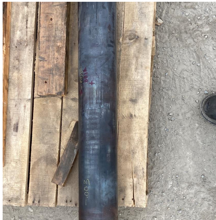
Figure 31. Views of oxide exfoliation on the CRV 2 basket (upper image) and the CRV 2 intercept valve stem with runout measurements (lower image).
