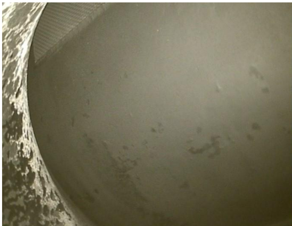
Figure 25. Borescope image of the HRH 2 manual stop / check valve disk (upper image) and CRV 1 basket (lower image) from the HRH 2 piping.
