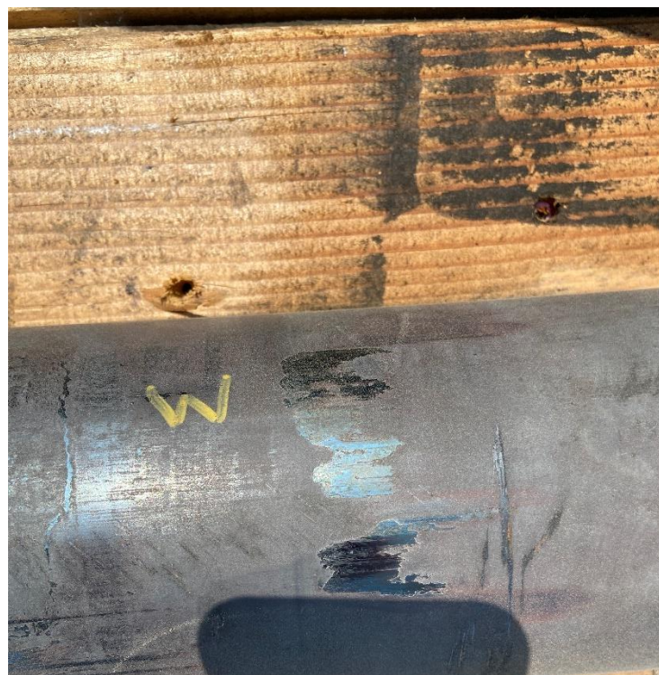
Figure 33. Views of the CRV 2 stop valve bushings (upper image) and stem witness marks (lower image).
