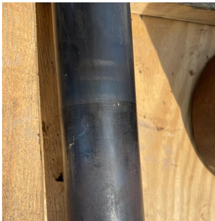
Figure 32. Views of the CRV 2 intercept valve stem with runout measurements and witness marks.
