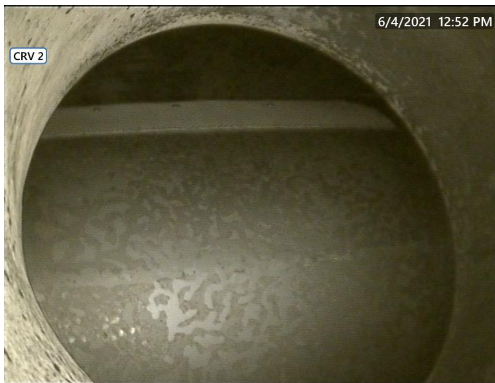
Figure 27. Borescope image of the HRH 1 piping showing oxide exfoliation (upper image) downstream of the manual stop / check valve and the CRV 2 basket (lower image).
