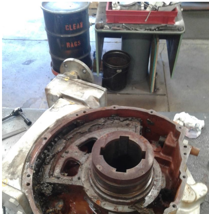
Figure 35. Images from the Bay Valves service center showing the HRSG 1 CRH stop valve (upper image) as received and disassembled gearbox (lower image).
