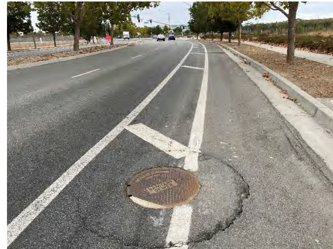
Photo 16: Looking east on Orchard Pkwy at sanitary sewer manhole (off site)- northeast perimeter of Property.
