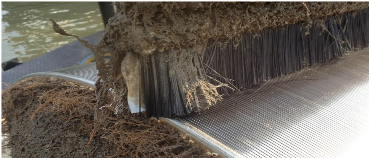
Figure 2-13: ISI mechanical brush-cleaned screen operating in Hudson River (Intake Screens, Inc. Report)
