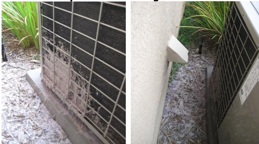
Figure 4-2: Noncompliant Condensing Unit Clearance from Dryer Vents
