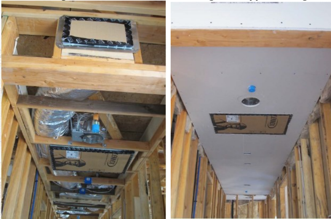
Figure 4-11: Ducts Routed Through a Dropped Ceiling
