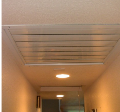
Figure 4-38: Whole-House Fan With Barometric Damper
