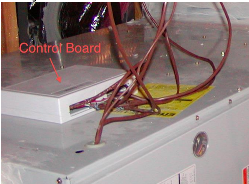
Figure 7: Photo of a cabinet-mounted control board.
