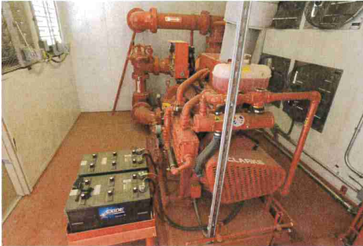
S-6 Emergency Fire Pump
