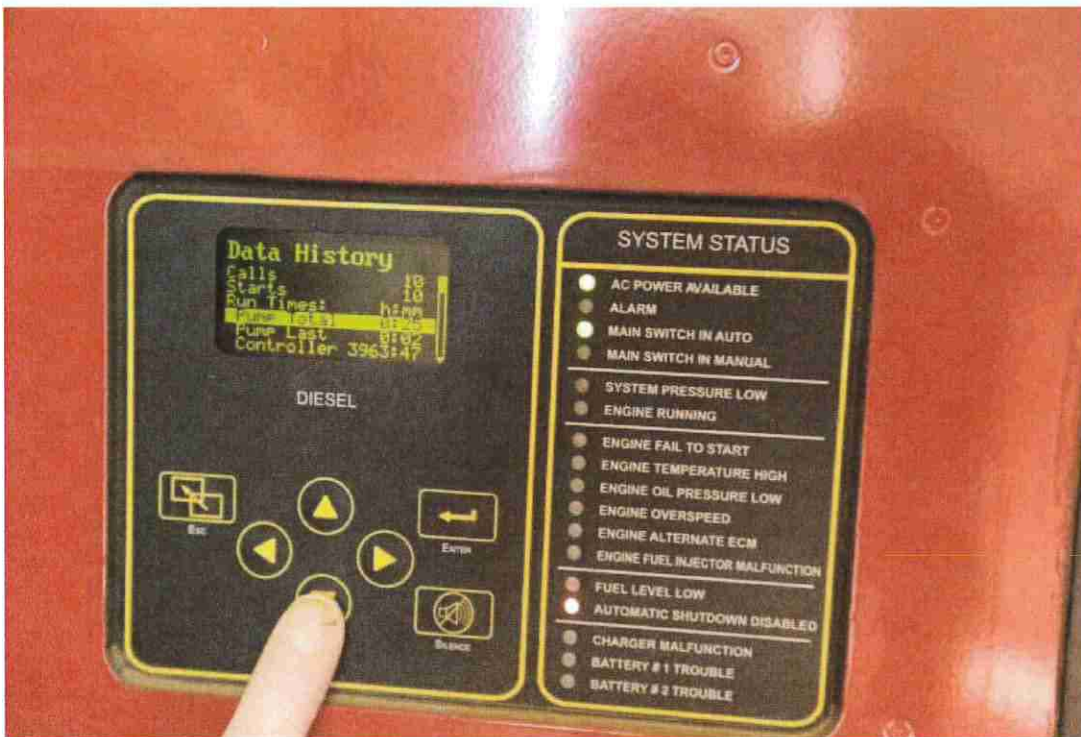
S-6 Controller, Showing Fire Pump Operating Hours
