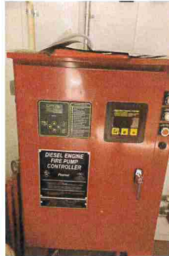
S-6 Control Unit
