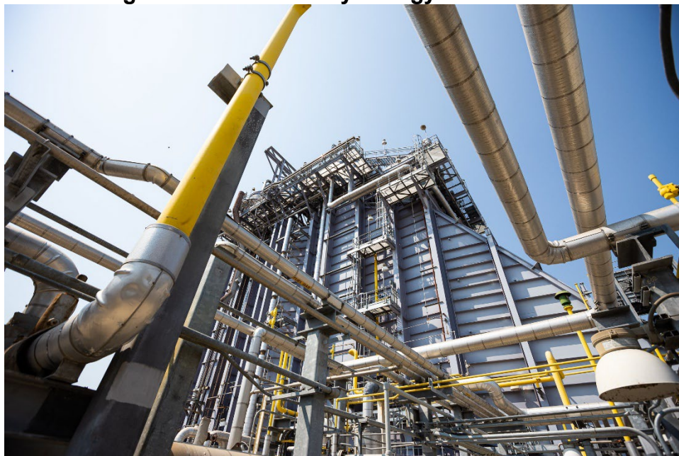
View of heat recovery steam generator from ground level
