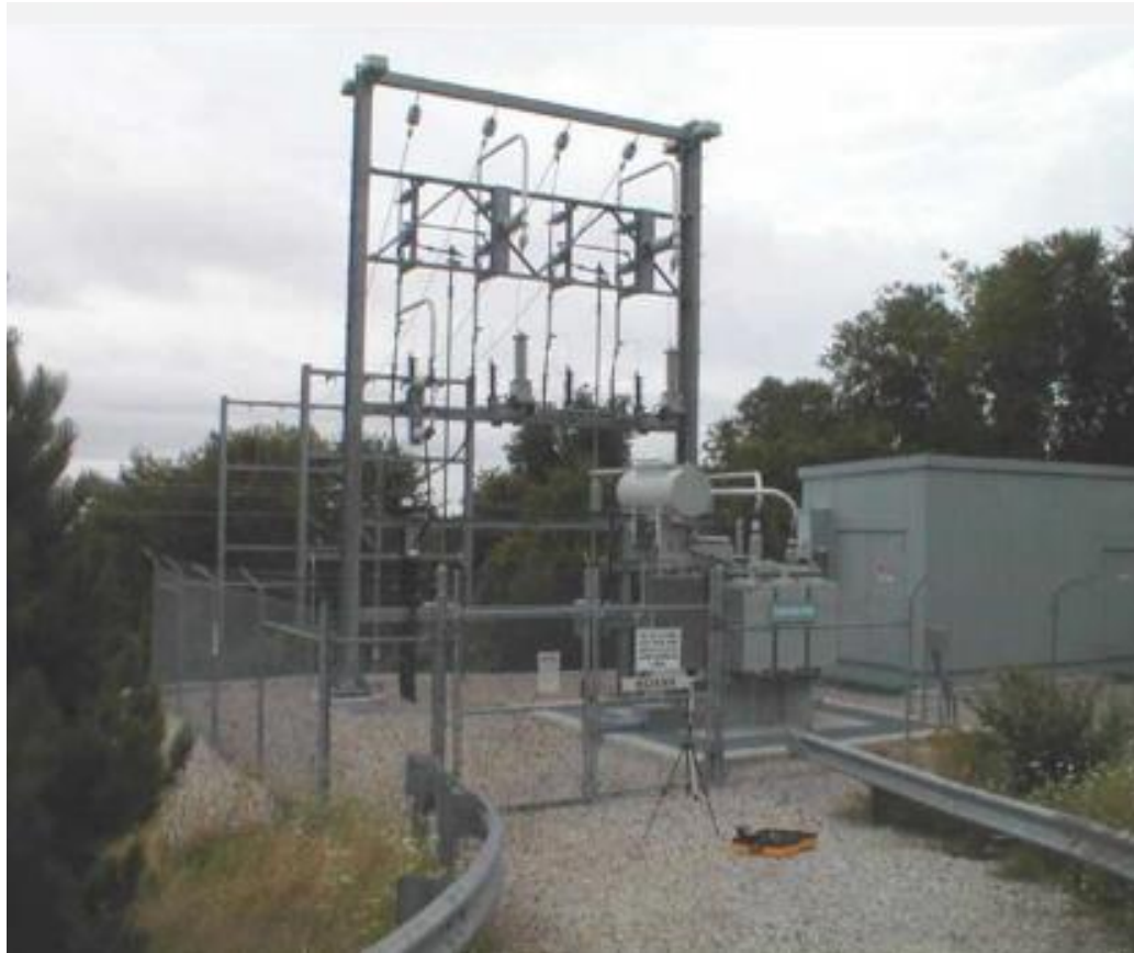
Paralleling Station - Amtrak Northeast Corridor
