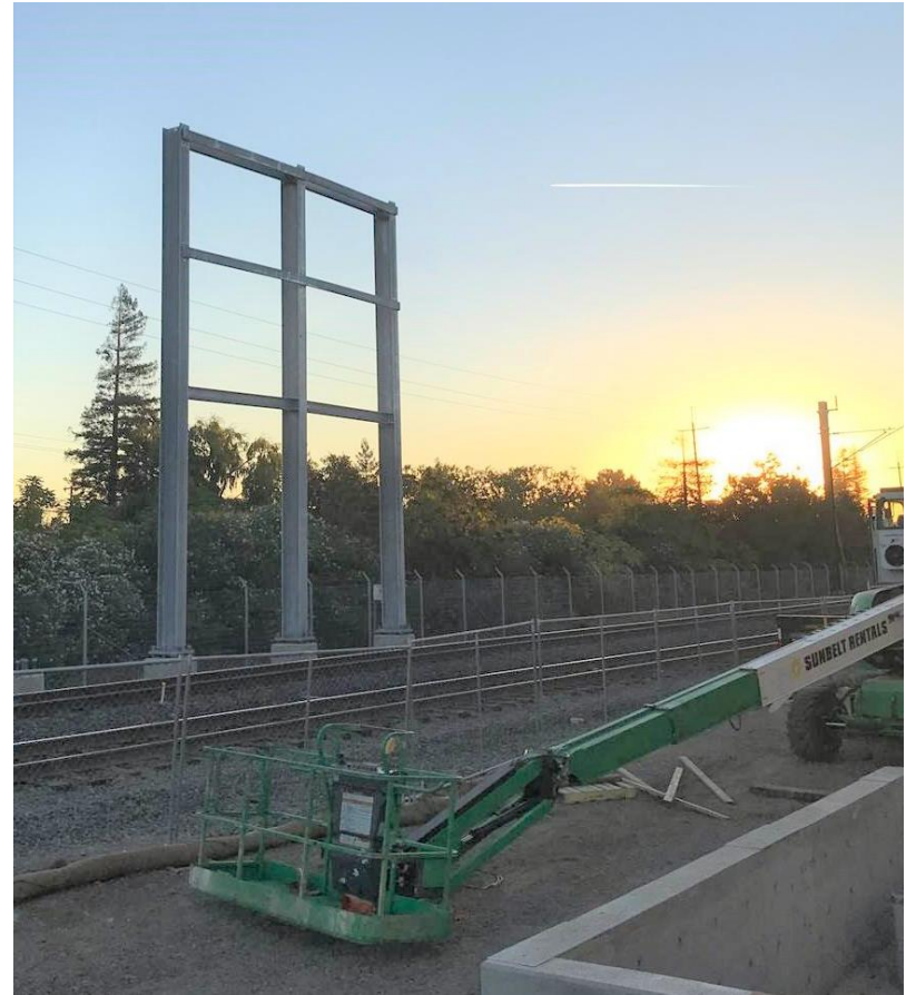
Strain Gantry – Palo Alto
