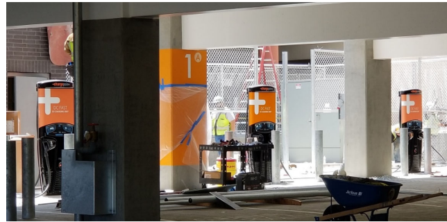
3 Charge Point FCDC in new parking structure E, 1st level
