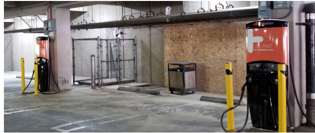
3 Charge Point FCDC in parking structure B, B level
