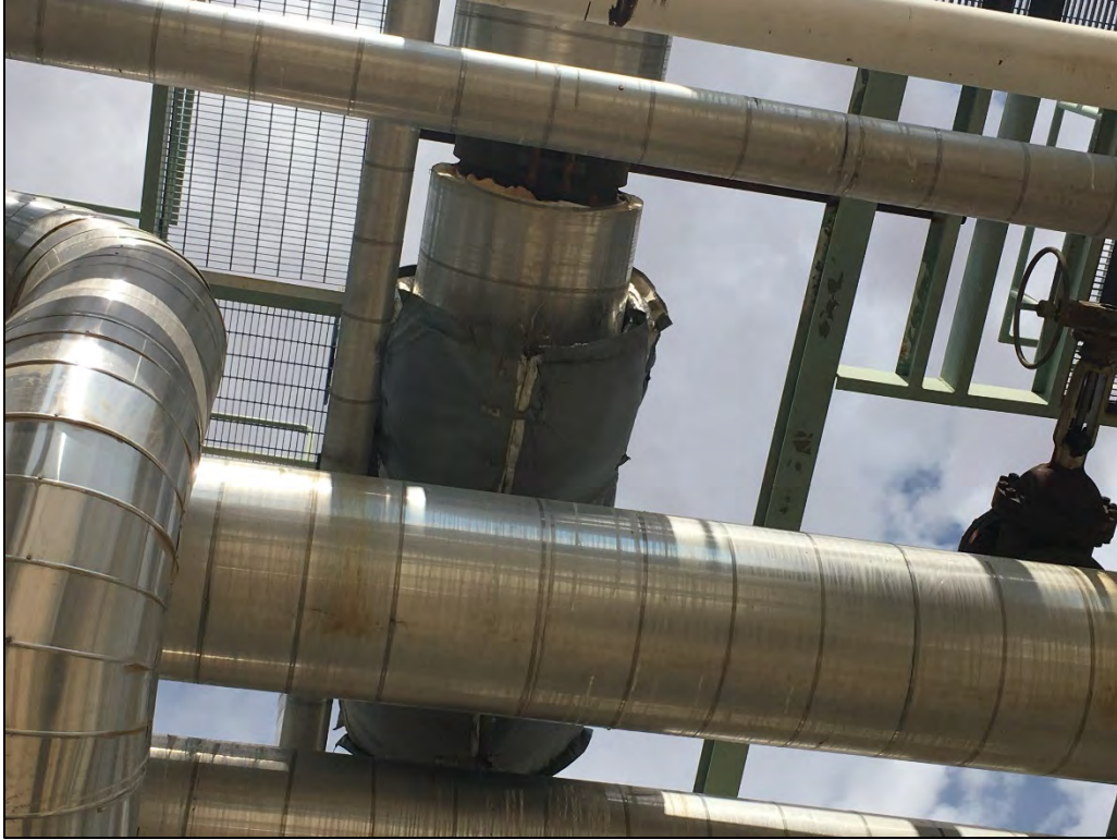
Photo 5: Underside view of inactive nest in pipe lining.
