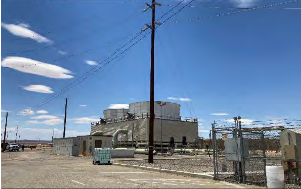
SEGSIV Cooling Towers
