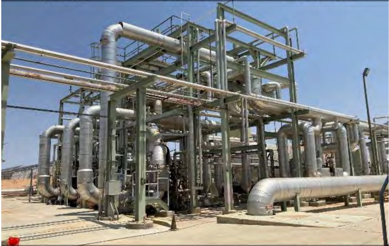
SEGSIV Power Block
