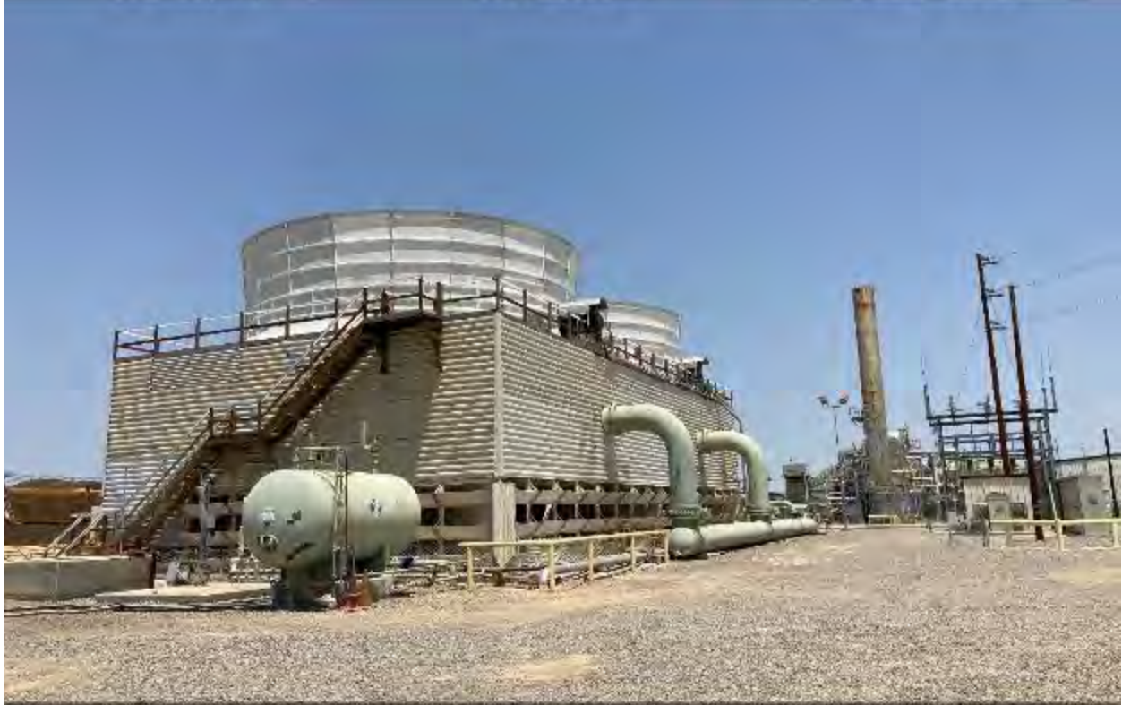
SEGSIV Cooling Towers
