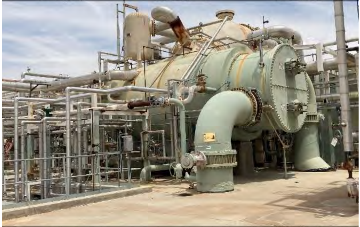
SEGSV Power Block
