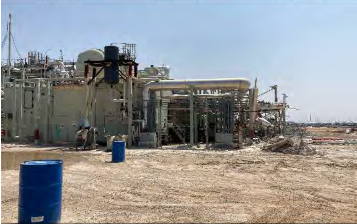
SEGSIII Power Block
