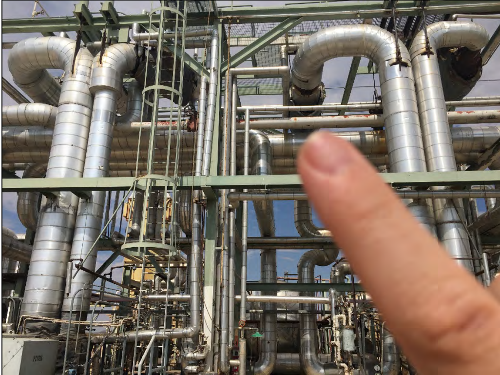
Photo 4: Old stick nest in pipe lining, inactive, likely common raven.
