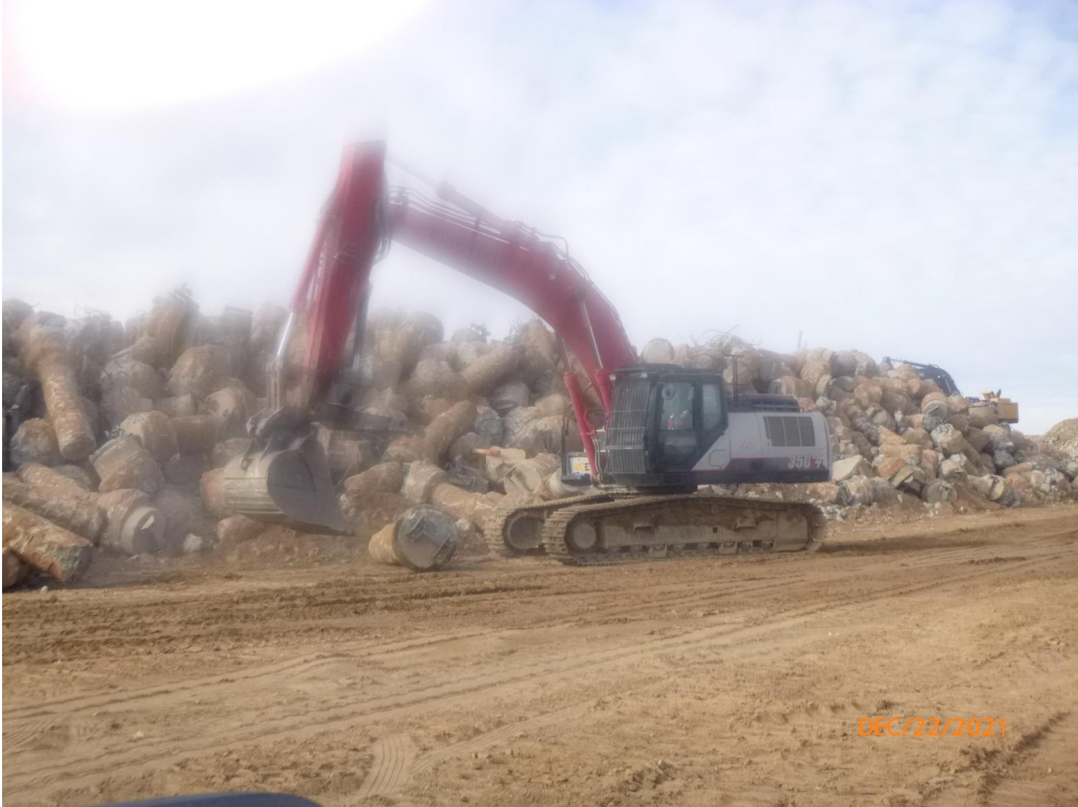
#10 SEGS Pier Concrete castings being crushed by equipment to remove steel embedment
