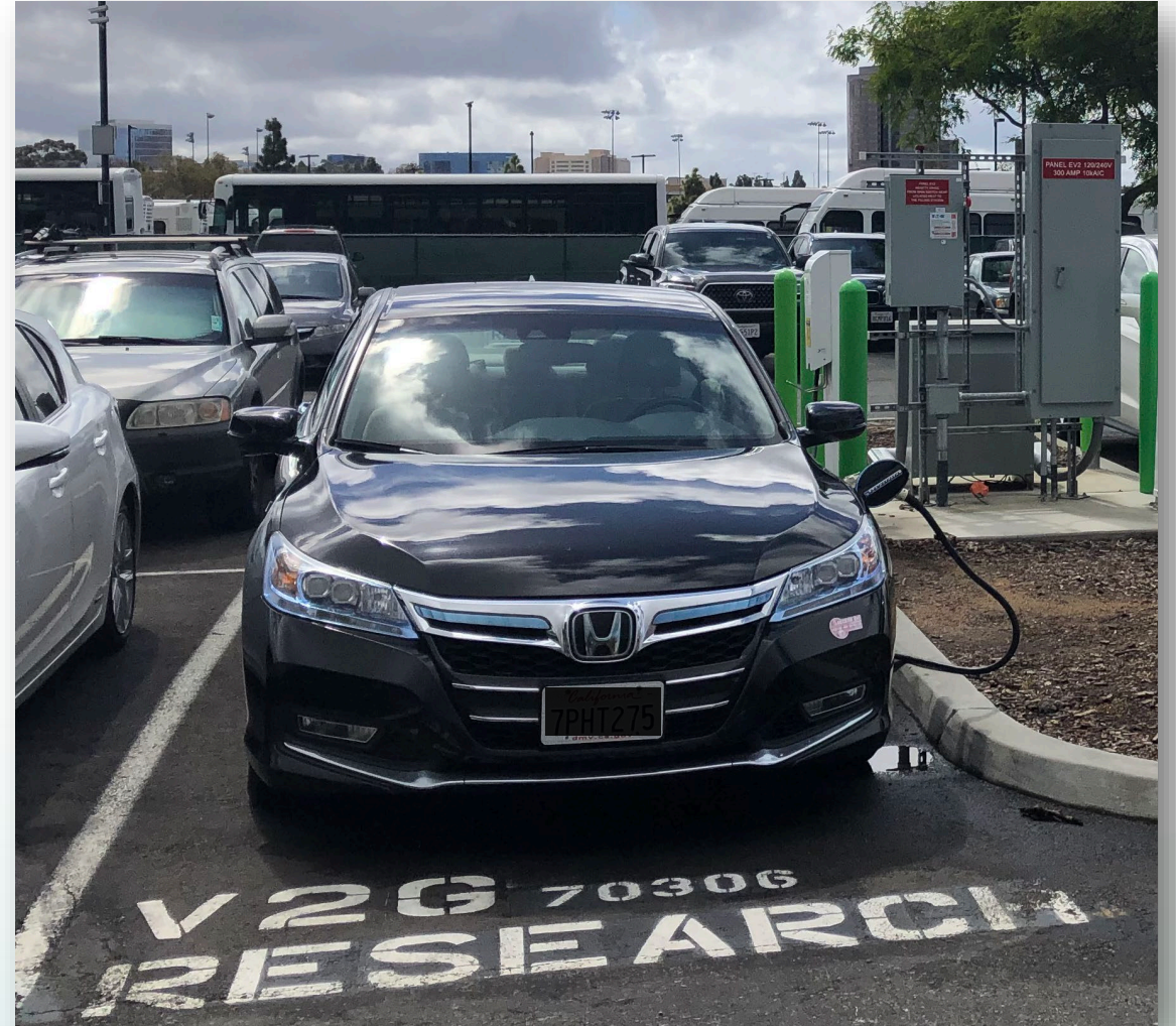
Bidirectional charging (source: Nuvve EPIC project EPC-16-061)
