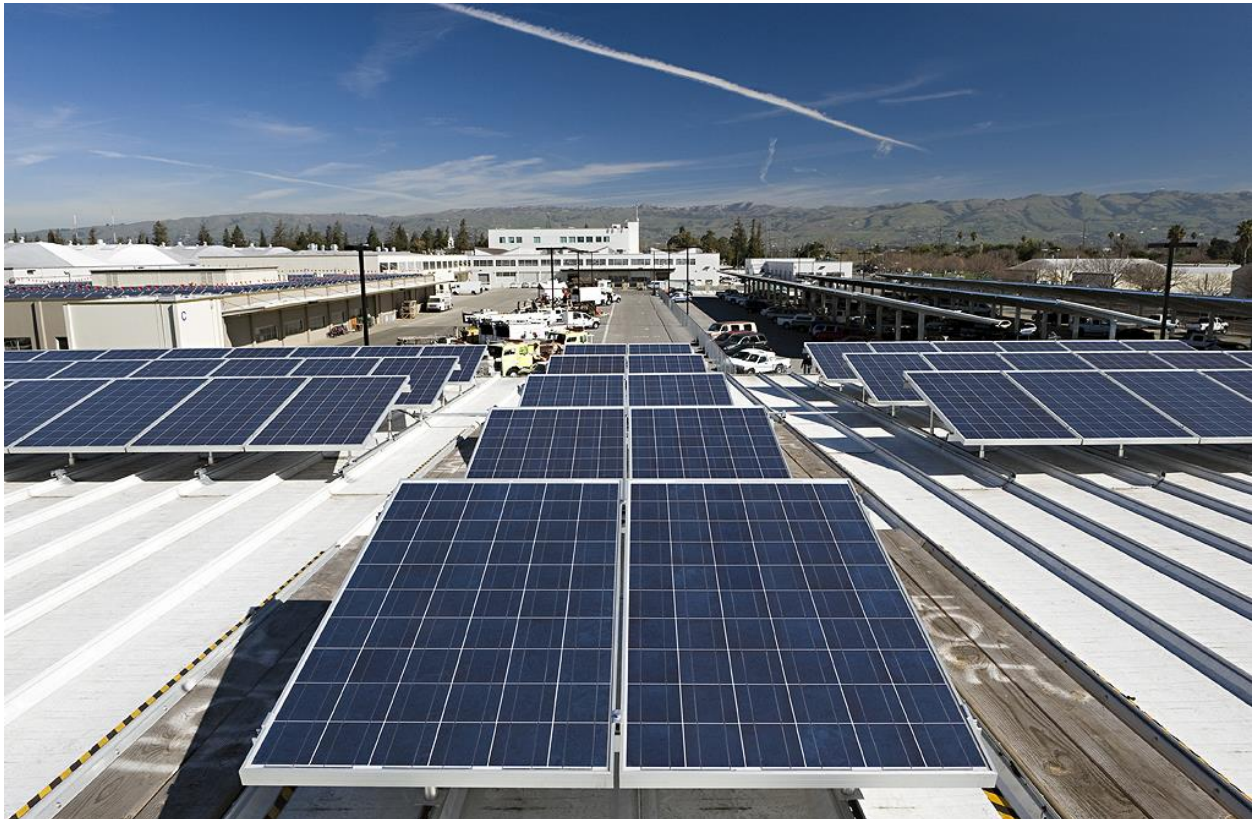
Solar installation at the Central Service Yard
