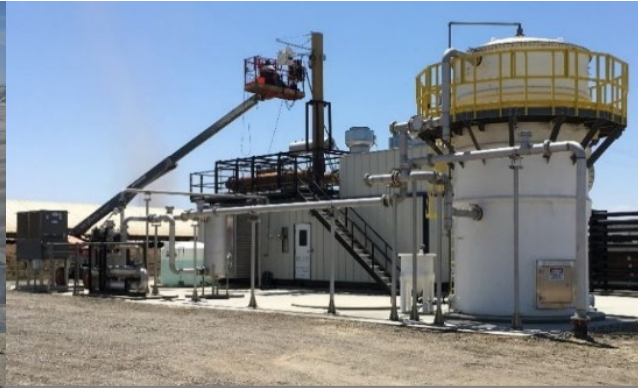
H2S Sponge scrubber (Biogas Storage Project)
