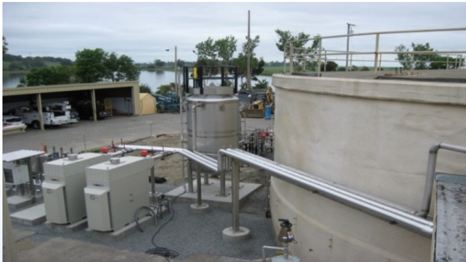
Photograph of microturbines, gas cleanup system and digester
