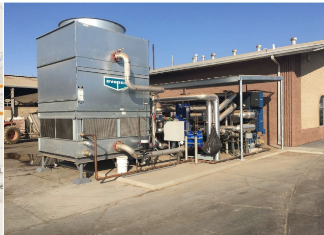
CHP Cooling Tower & Chiller (CHP Project)
