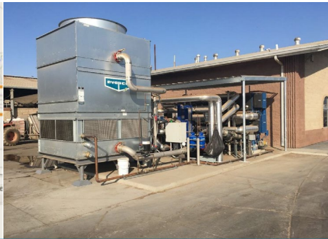
CHP Cooling Tower & Chiller (CHP Project)
