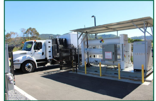
Time-fill RNG Station ( top picture ) and Fast-fill CNG station ( bottom picture ).
