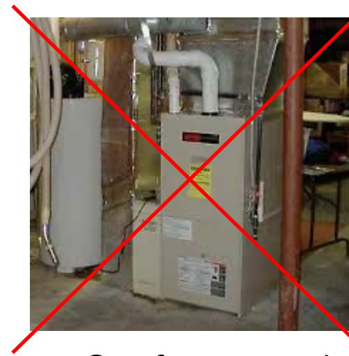
Gas furnace and water heater
