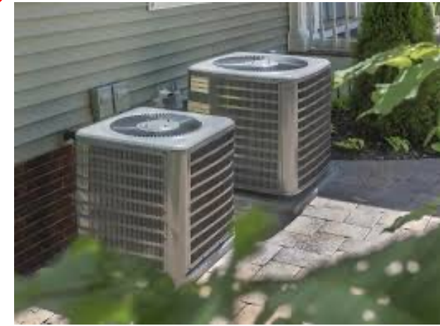
Heat pump heating and cooling
