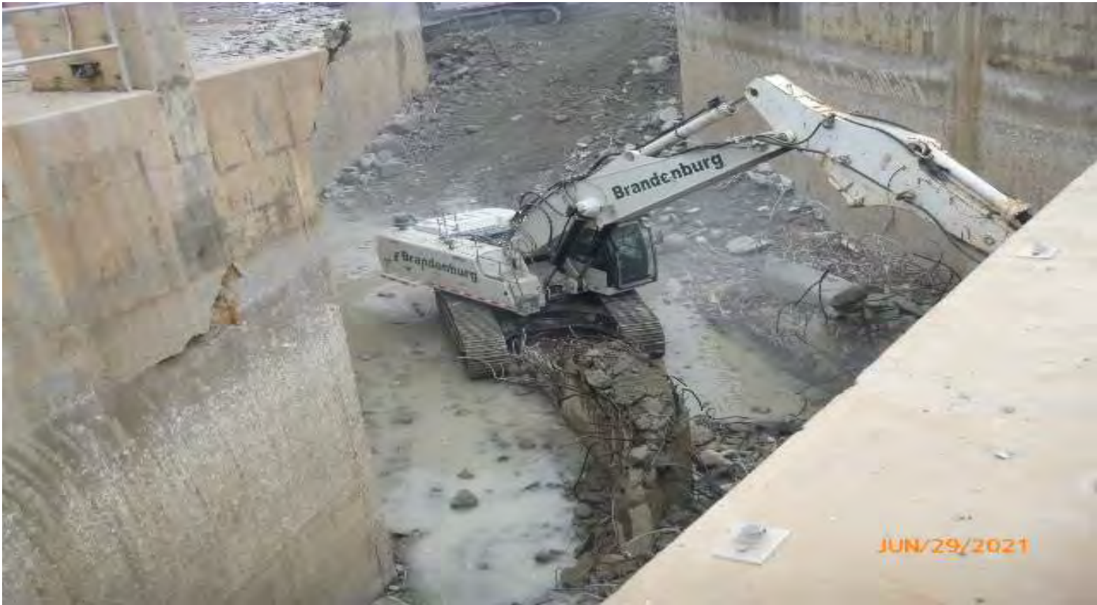
Photo #13: Demo point of excavator breaking center walls in water channel areas
