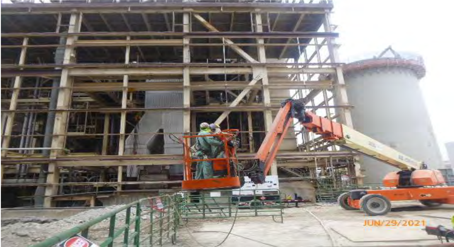
Photo #4: Transmission Bay area looking north, stack under active demo on right.
