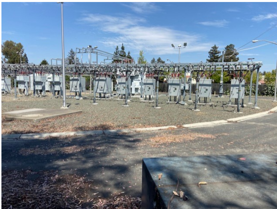
Photograph 6. Overview of substation transformers; facing east.
