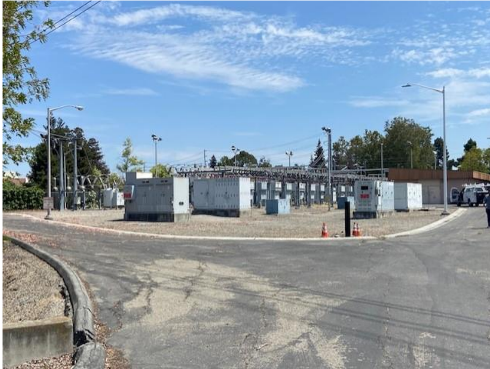
Photograph 5. Overview of substation, yard, equipment, and building; facing south.
