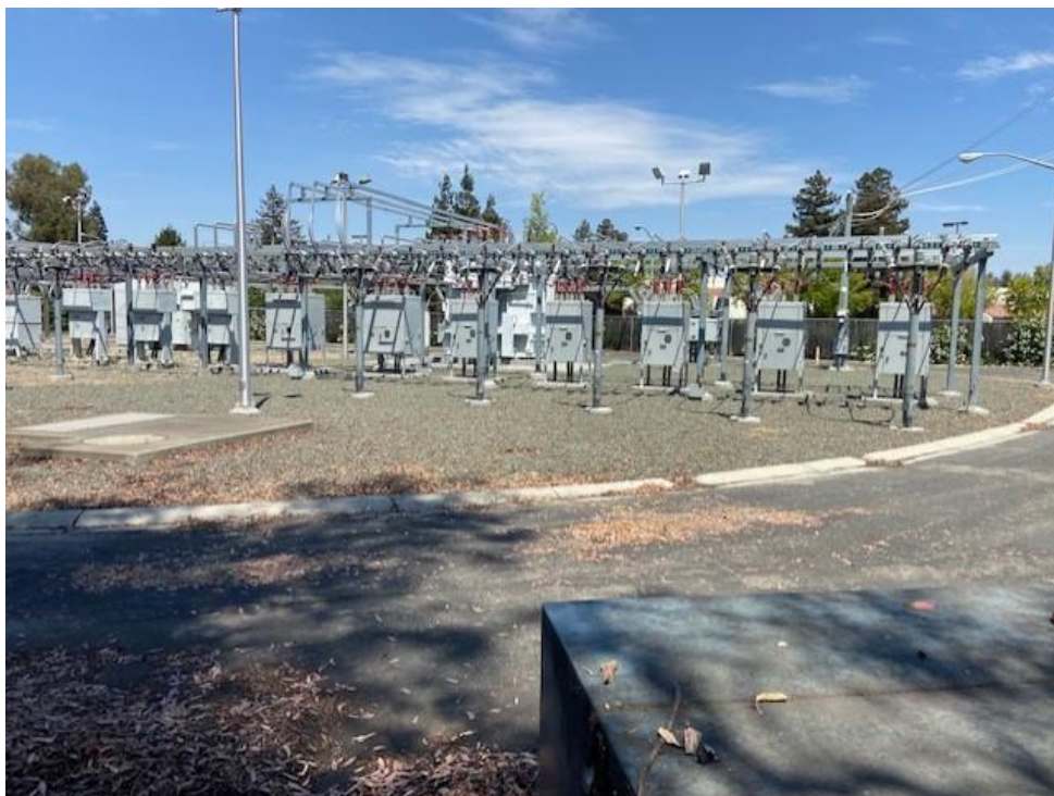
Photograph 6. Overview of substation transformers; facing east.
