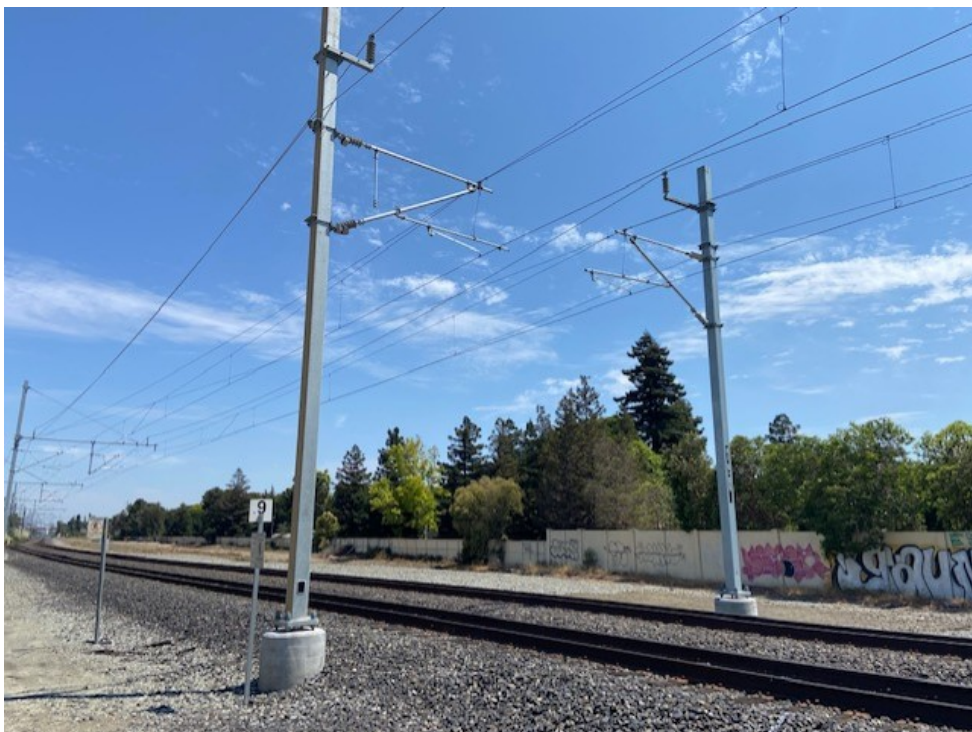
Photograph 4. Detail view Caltrain electrified towers and wires; facing southeast.
