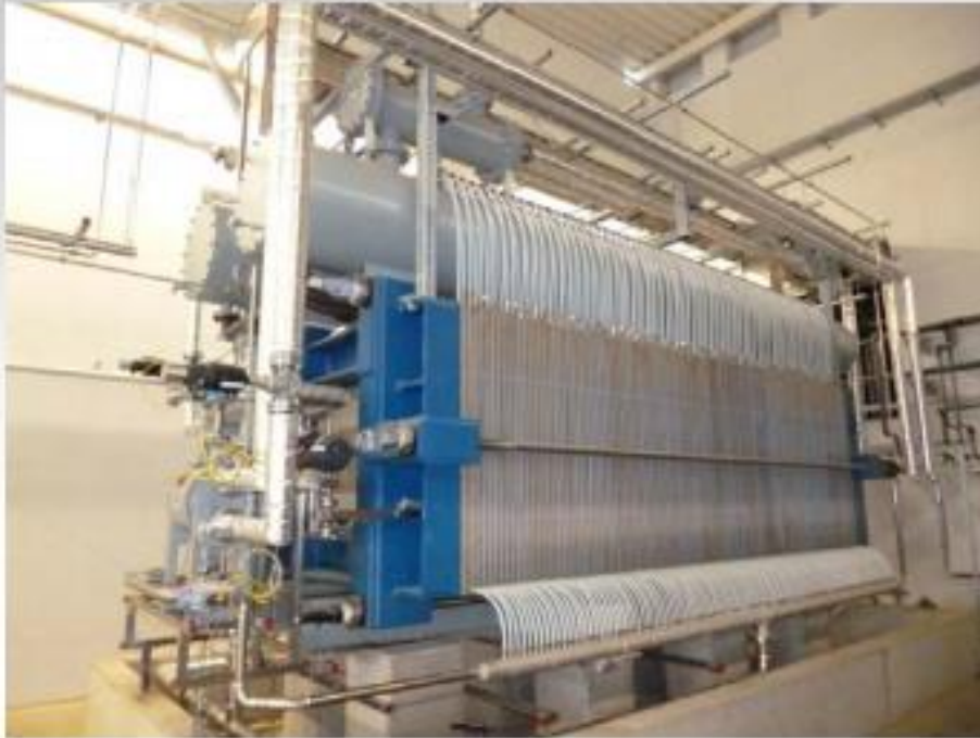
Electrolyzers (3 x 2 MW)
