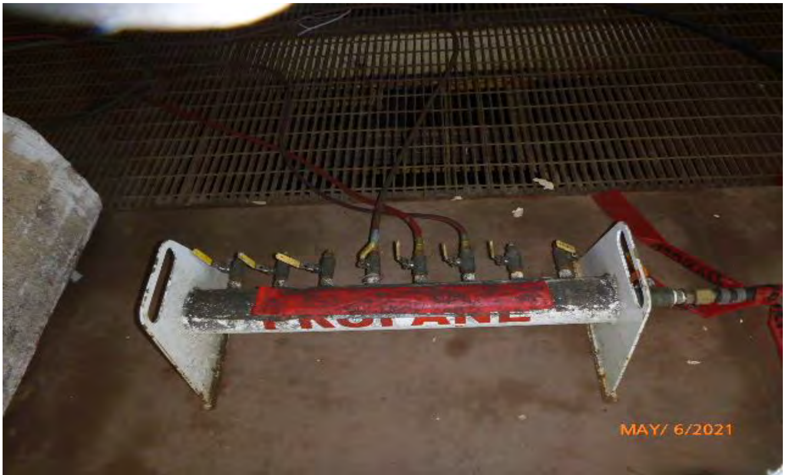
Photo #3: Propane Gas Manifold for cutting of metal structure
