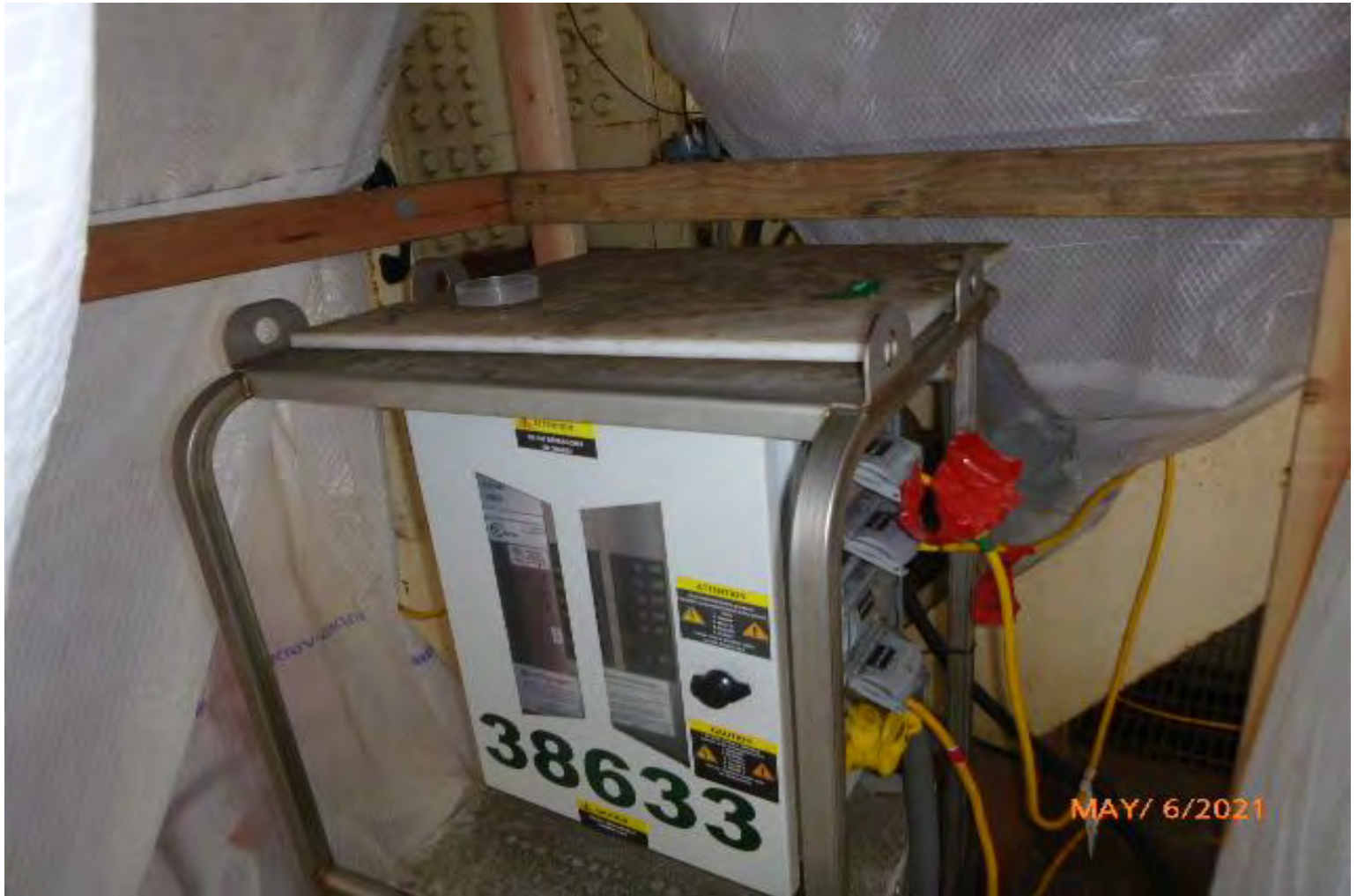
Photo #2: Temporary Power and Cords organized and supported.
