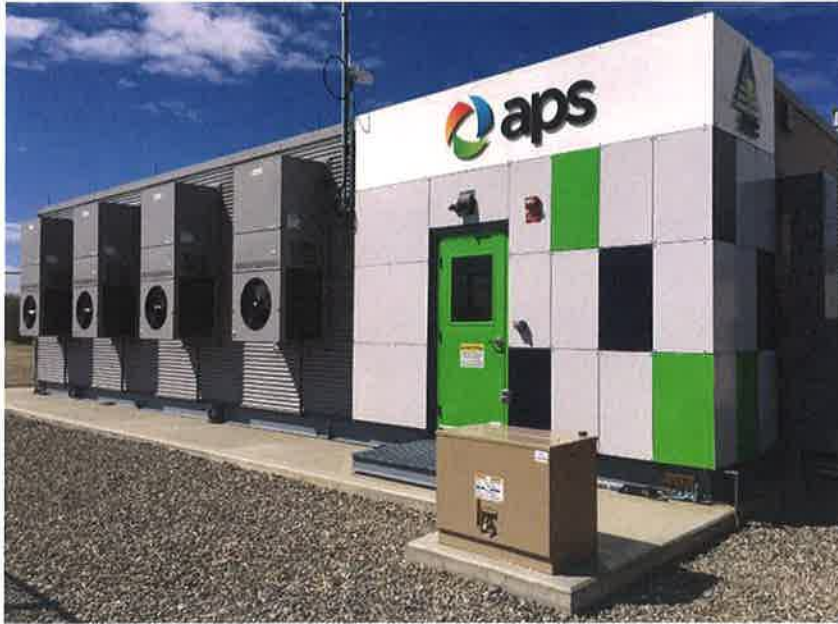
Arizona Public Service's 2-MW battery storage project in Surprise, Ariz., before a fire in April took it offline.
