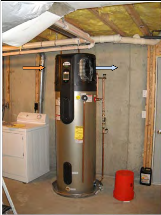
Figure 7. HPWH installed with adequate clearances
