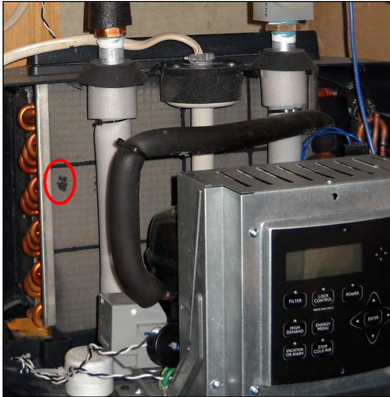
Figure 15. Dirty filter: finger rubbed against filter to show accumulation of dirt
