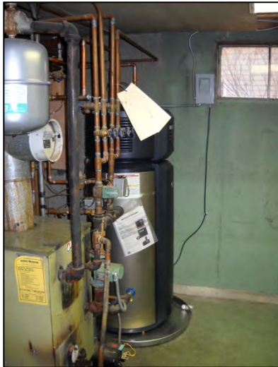
Figure 9. HPWH installed in boiler room
