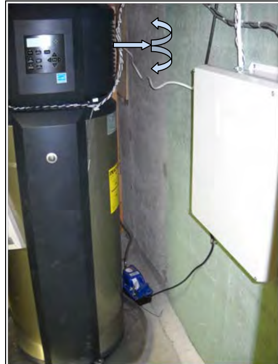
Figure 8. Improper HPWH with air discharge facing wall
