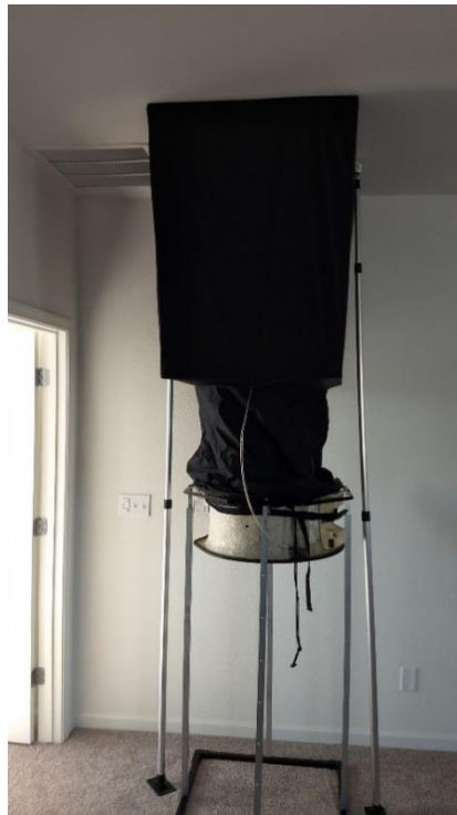
Figure 6: The QuietCool PFH installed
