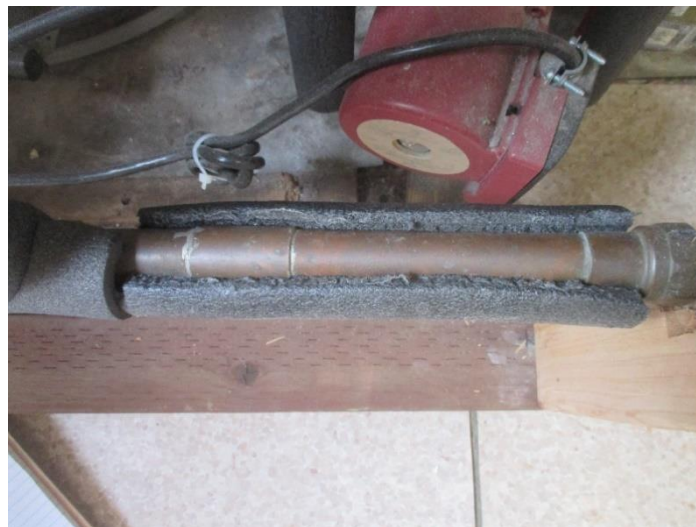
Figure 15: Poorly installed insulation.
