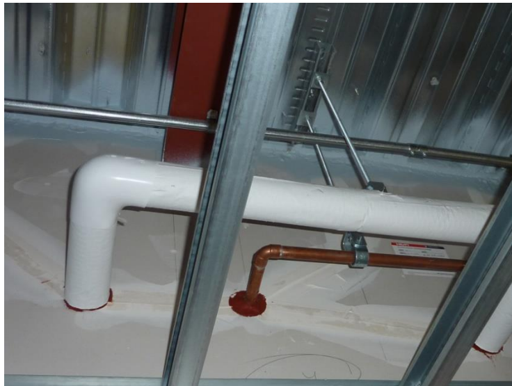
Figure 13: Metal hangers not thermally isolated from metal pipe.
