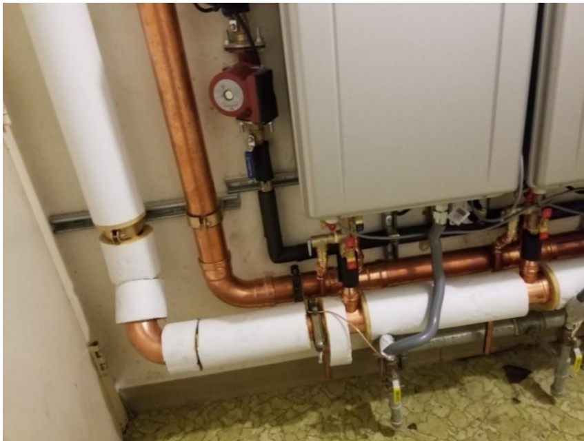
Figure 2: Field observation punch list photo showing missing pipe insulation.
