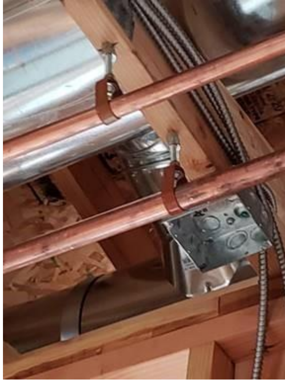
Figure 12: Metal hangers not thermally isolated from metal pipe.
