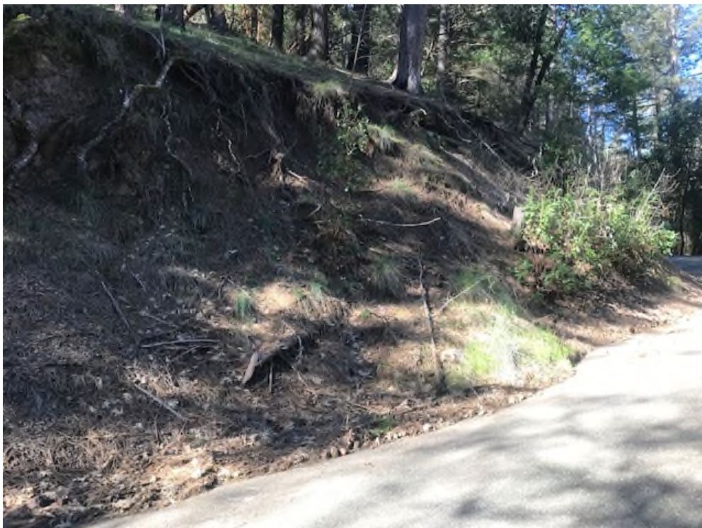
Upper re-seeded section of High Valley Road
