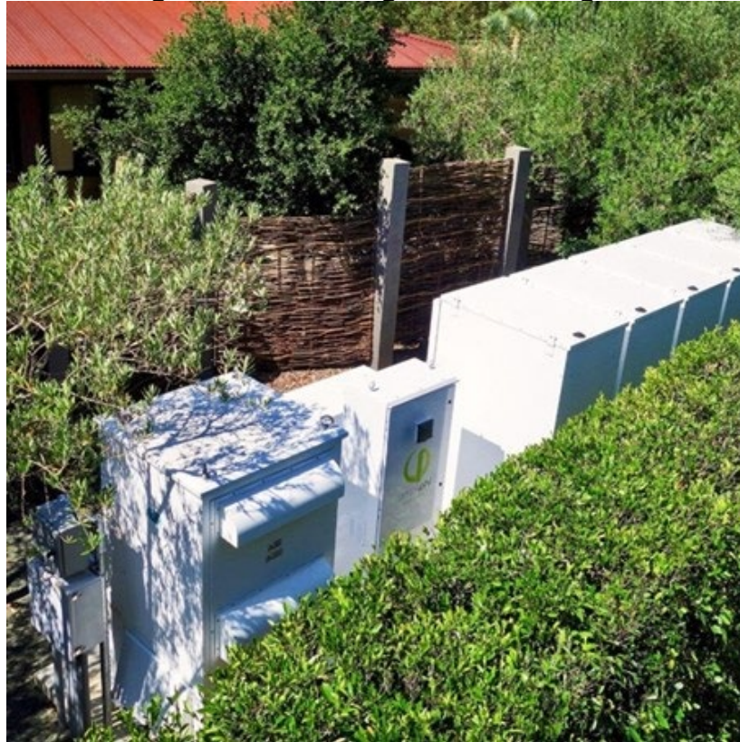
Figure 4: Stone Edge Farm Microgrid
