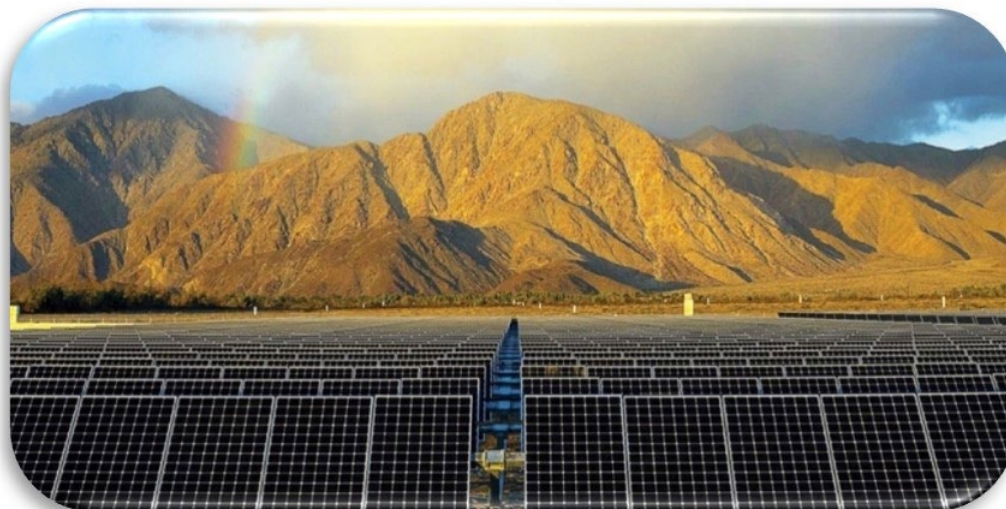
Figure 5: Borrego Springs Microgrid
