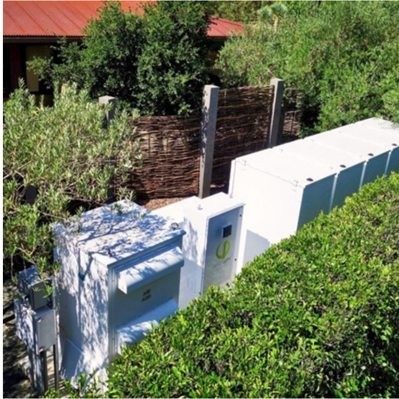
Figure 4: Stone Edge Farm Microgrid
