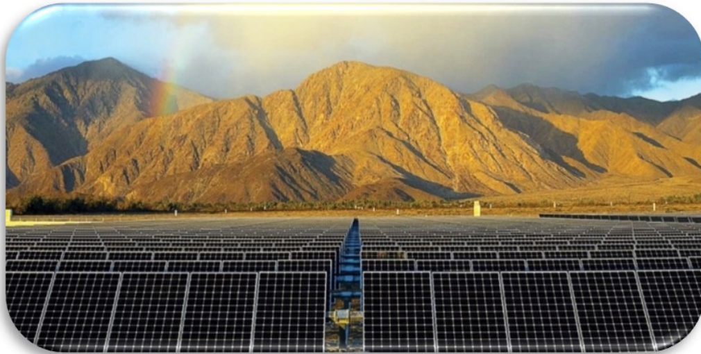
Figure 5: Borrego Springs Microgrid
