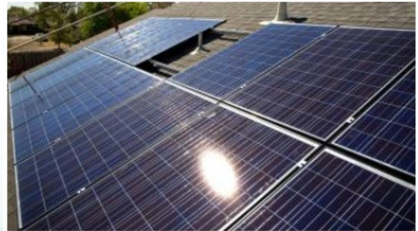
Photo above shows solar PV on roof.
