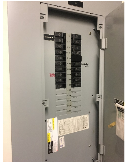
200 amp panel with 10 breaker spaces available.
