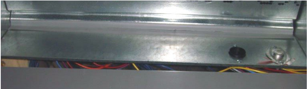
Figure 1: Unsealed economizer perimeter gap for a 3-ton RTU (Mowris 2016)
