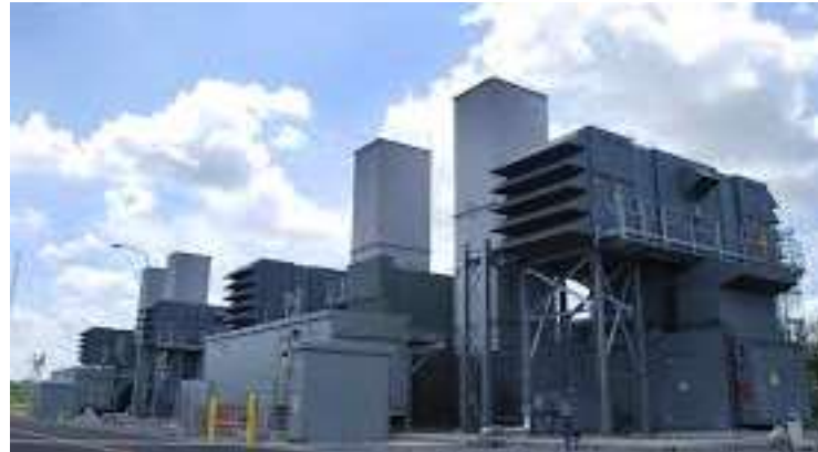
Peaking Gas Turbine
