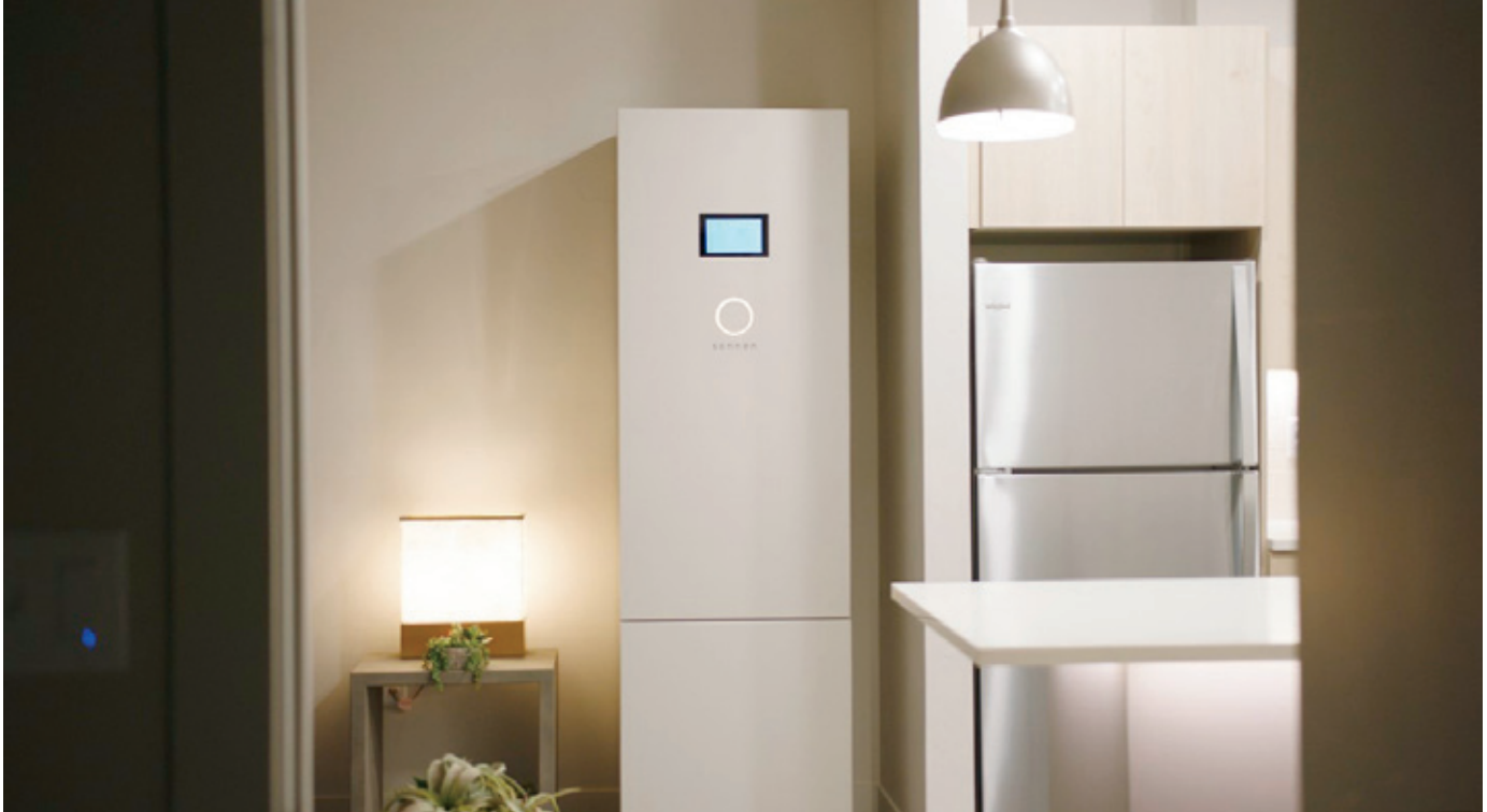
Sonnen battery storage system in an apartment at Soleil Lofts in Utah.
