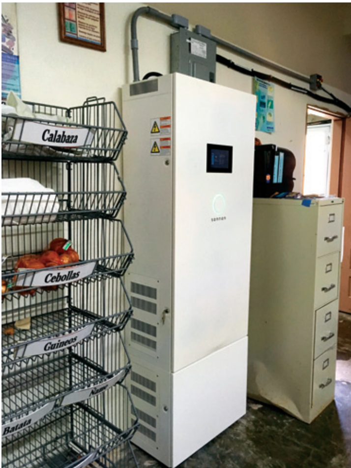
Residential and small commercial battery systems, like this 14-kilowatt-hour sonnen eco 14 battery at a remote school in Orcovis, Puerto Rico, tend to have an average installed cost between $800 to $1,000 per kilowatt-hour.
