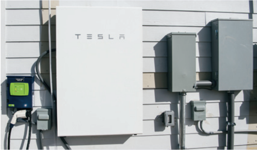
Tesla residential battery system.
