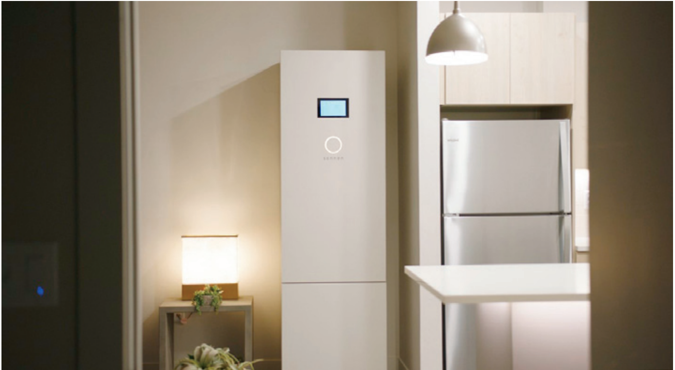
Sonnen battery storage system in an apartment at Soleil Lofts in Utah.
