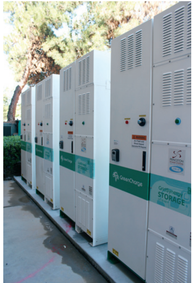
Battery systems in the 100 kilowatt-hour to 500 kilowatt-hour range, such as this system at a Safeway supermarket in San Jose, CA, typically cost less than smaller systems, around the $600 to $800 per kilowatt-hour range.
