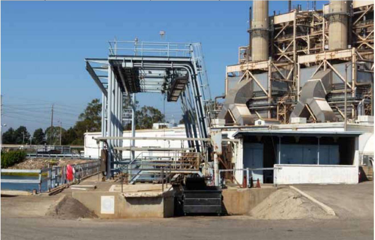
Units 3 and 4 Screen well at intake, view looking northwest. North intake channel is visible on the far left; Units 1 and 2 are on the right.
