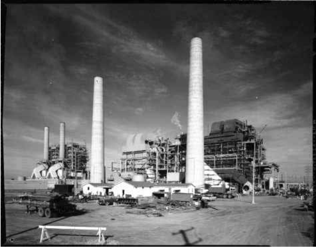
Units 3 and 4, view looking northwest, December 21, 1961. Units are under construction. Unit 3 is in middle of photo, Unit 4 is on the right. Units 1 and 2 are visible on the far left.
