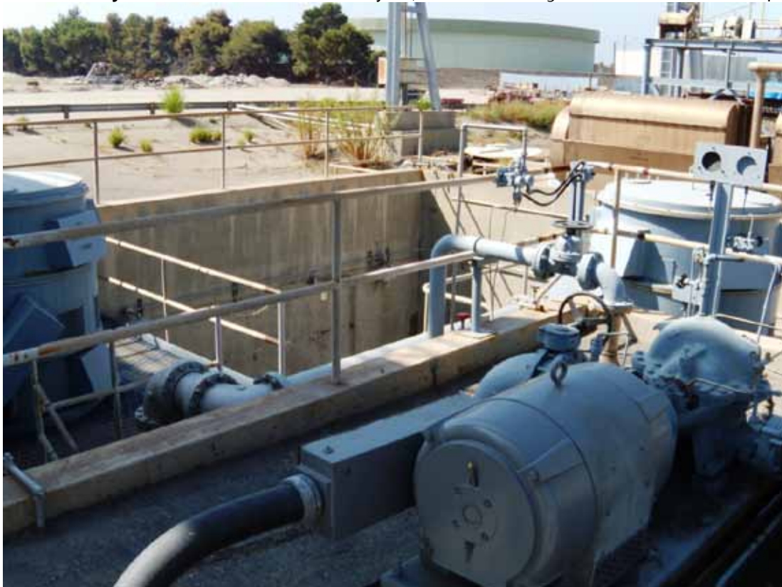
Units 5 and 6 Circulating Pumps at intake, view looking southwest
