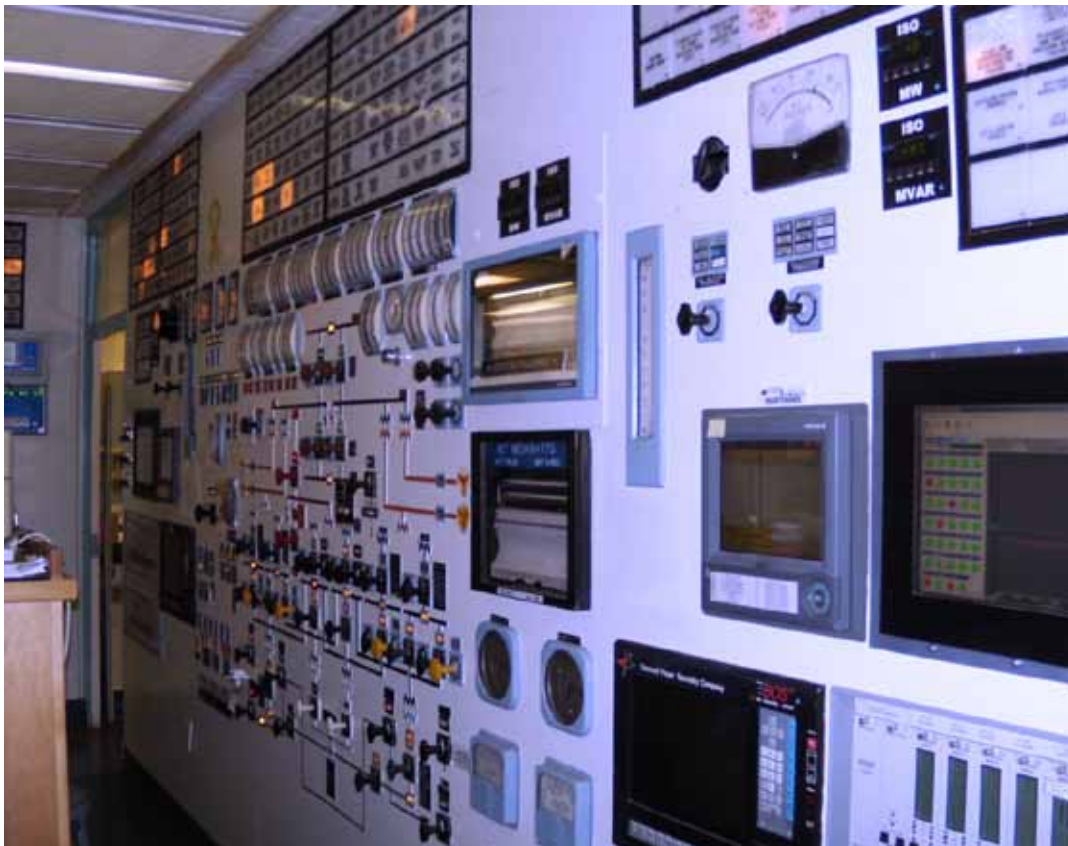
Interior view - control panel in control room for Units 5 and 6.
