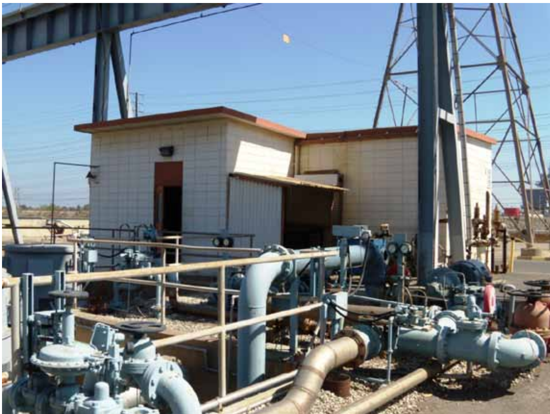
Circulating Pump Control House for Units 5 and 6, view looking northeast
