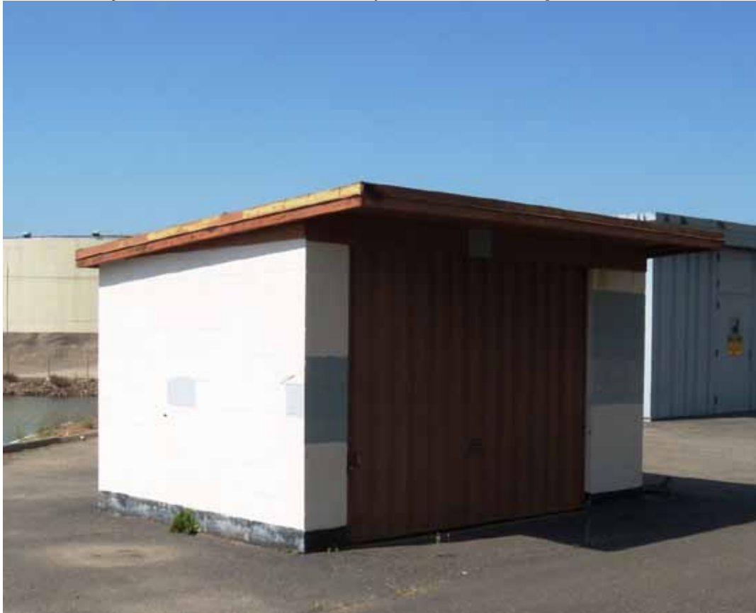
Units 5 and 6 west side hose house, view looking southwest
