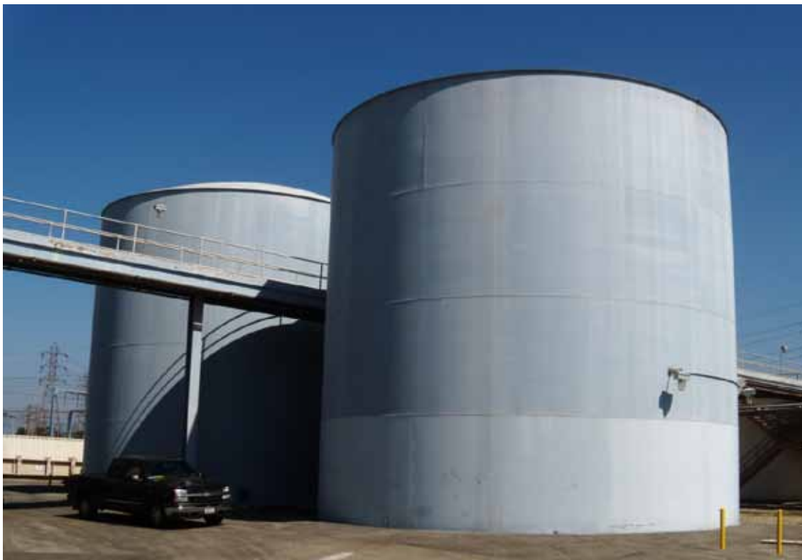
Units 3 and 4 Distilled water tanks, view looking northeast.
