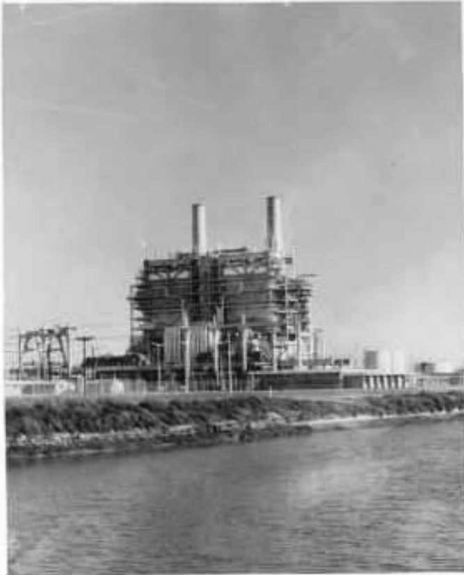
Units 1 and 2, view looking southeast, September 1958. (Photo from the Edison Archive. Courtesy of The Huntington Library, San Marino, CA)
