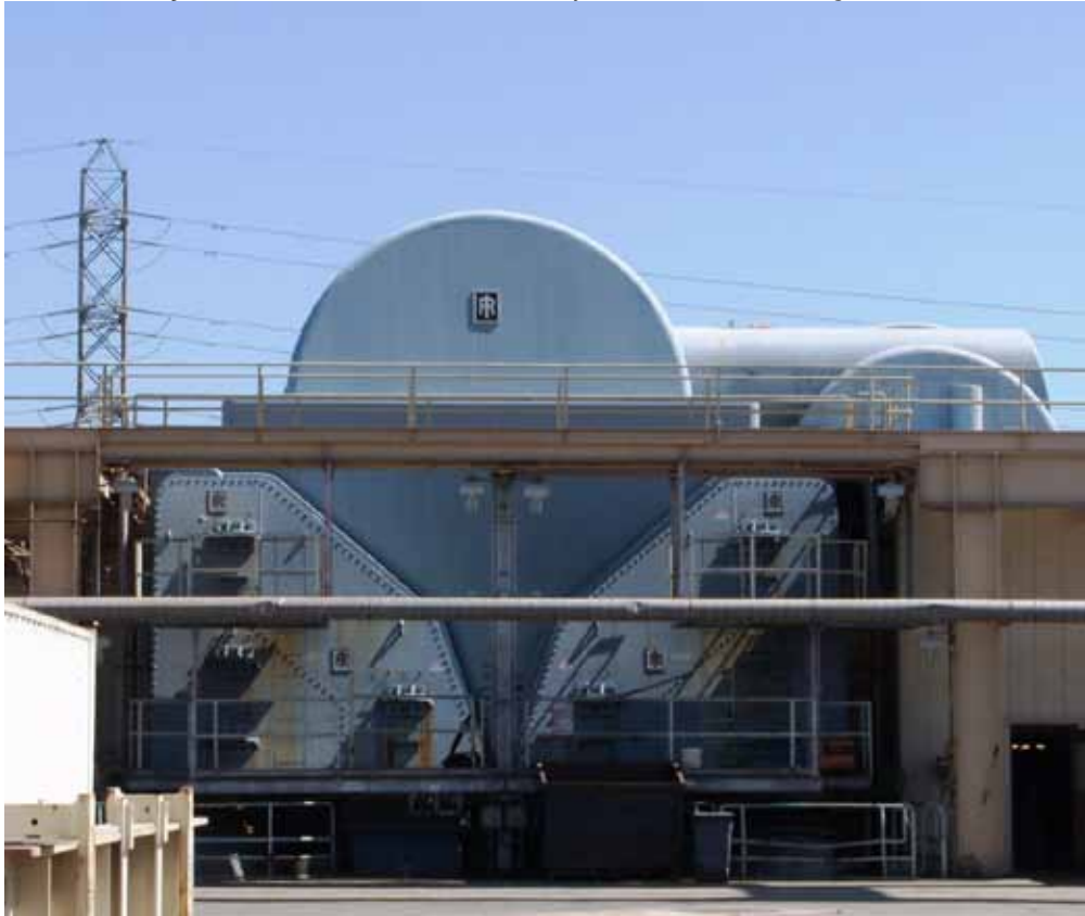
Unit 3 Ingersoll-Rand condenser, view looking east.
