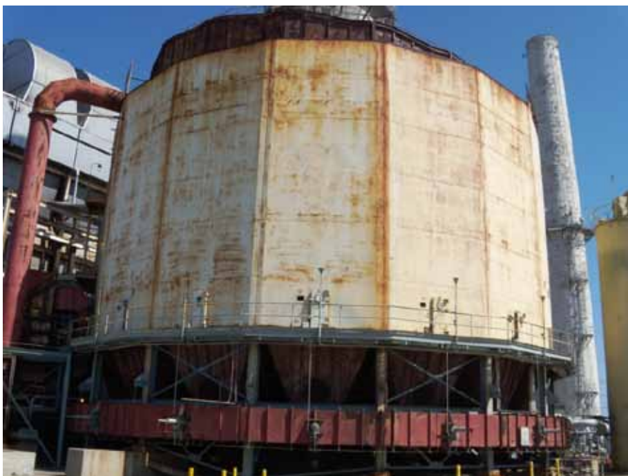
Unit 3 bag house, view looking northeast. Unit 4 stack is visible on the right.
