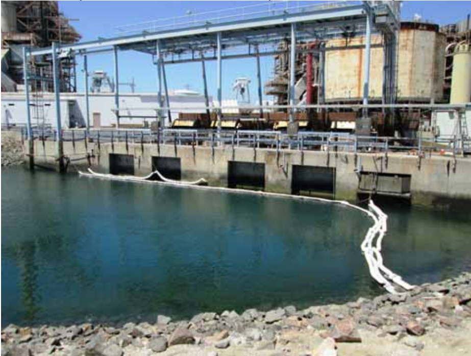
North intake channel – view to northeast of intake structure for Units 3 and 4
