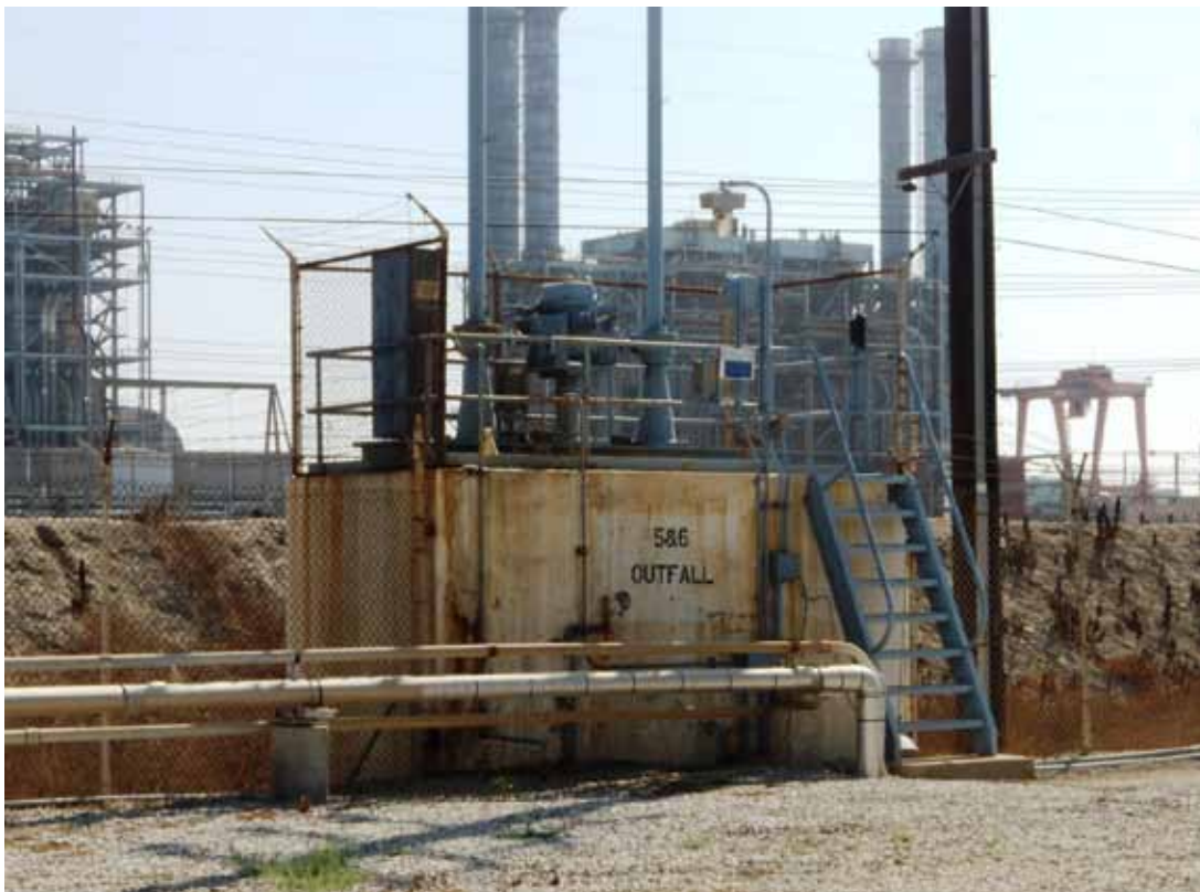
Outfall gates for Units 5 and 6, view looking southeast
