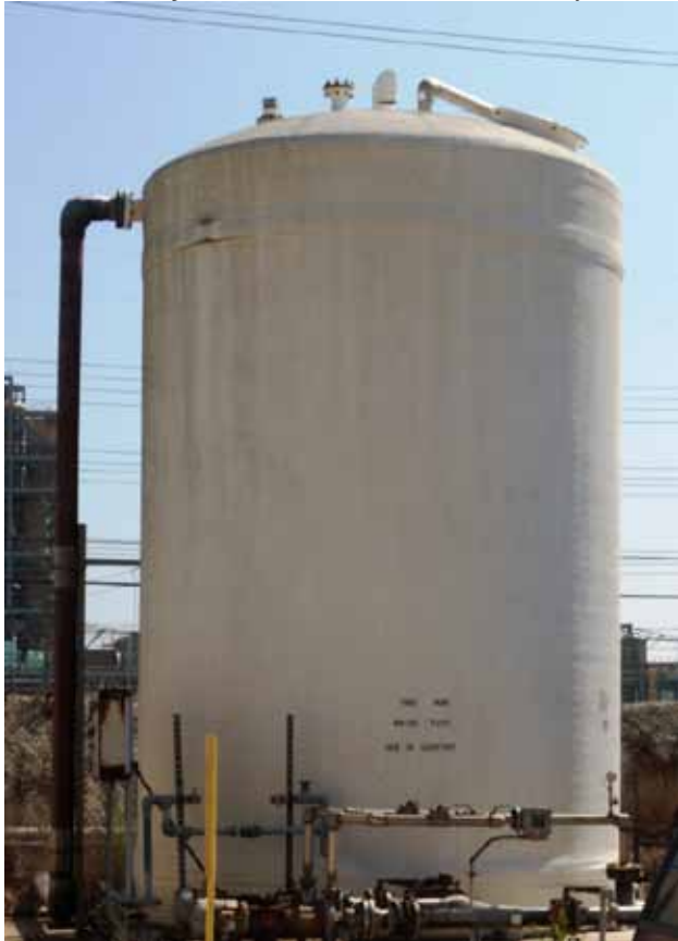
Brine tank for Units 5 and 6, view looking east.
