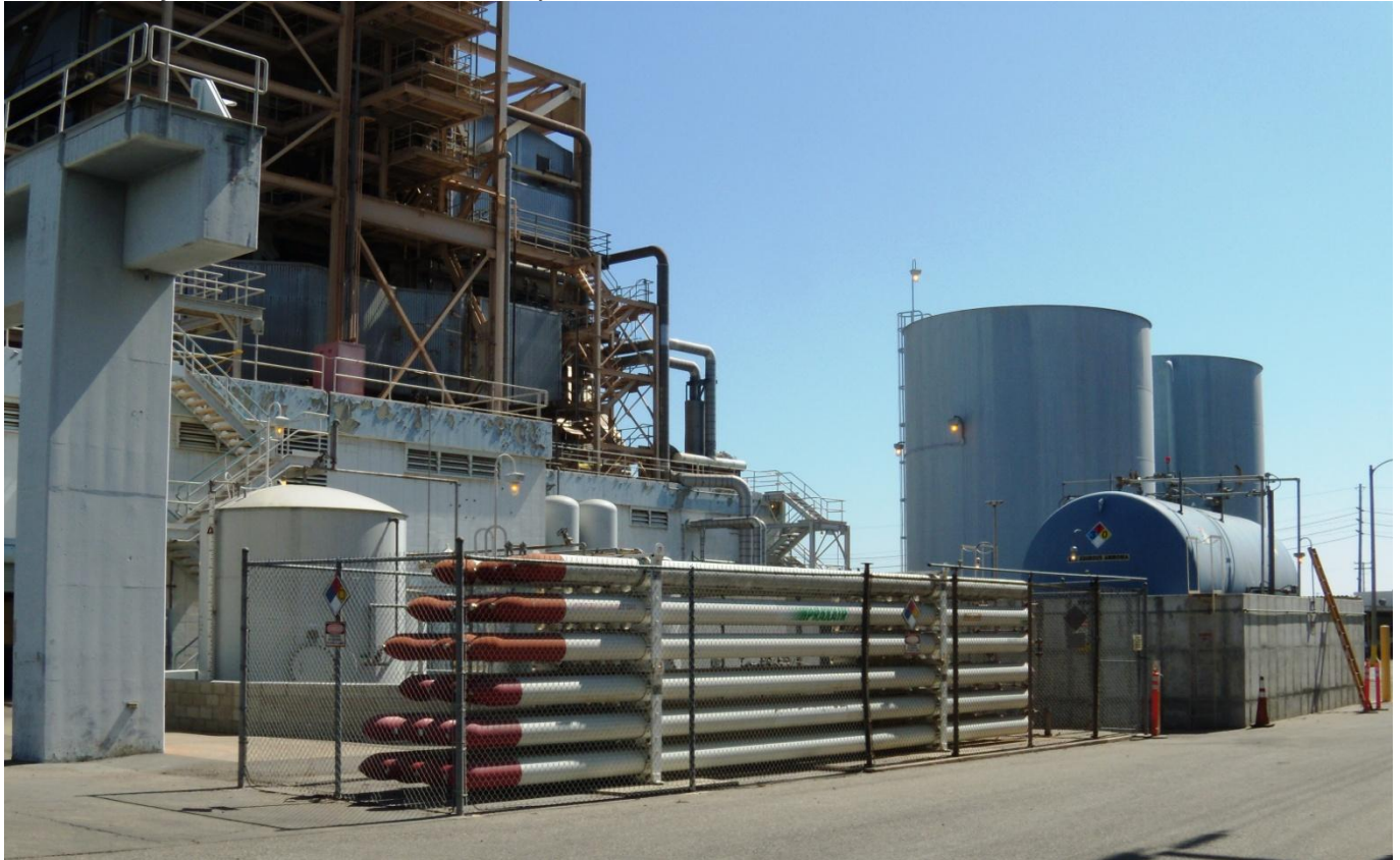
Unit 1 storage tanks (hydrogen, aqueous ammonia, and demineralized water), view looking southeast.
