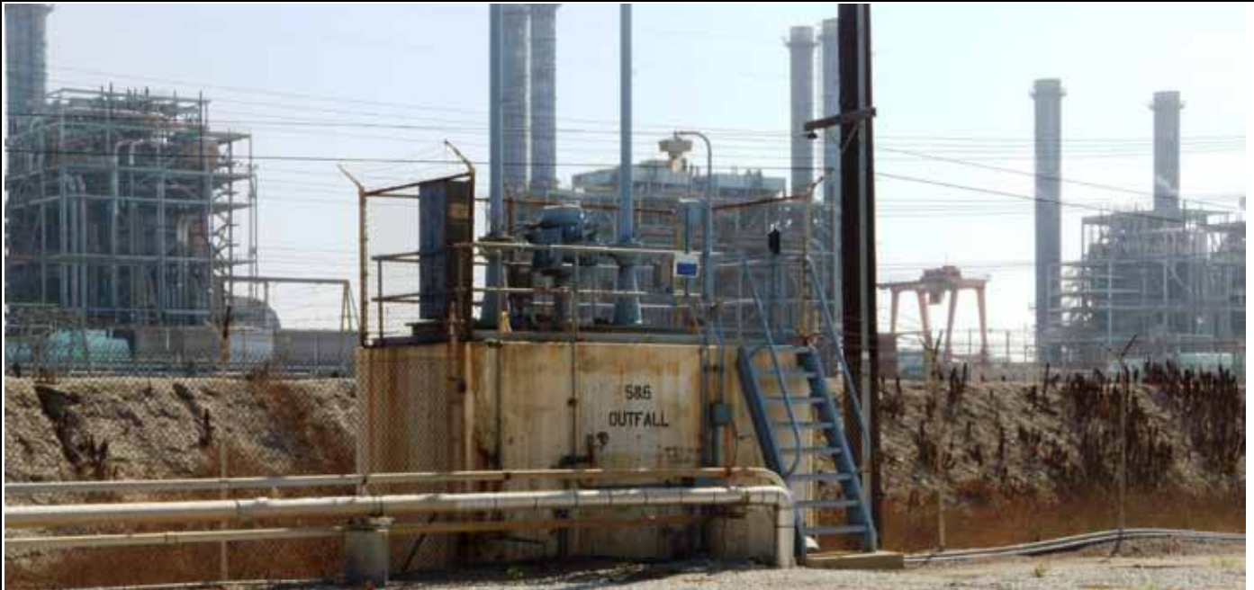
View looking southeast from AES Alamitos at outfall for units 5 & 6 and west side of west bank levee. September 2011.
