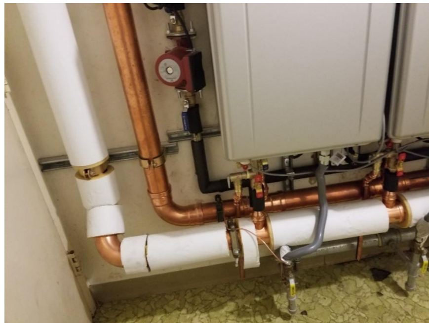
Figure 11: Uninsulated fittings and valves.
