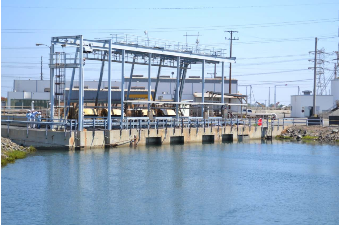
Alamos Energy Center. Photo of existing facilities, view facing east.
