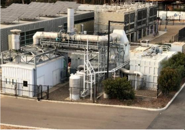
Figure 2: FCE SureSource 3000 system at UCSD campus in La Jolla
