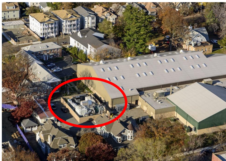
Figure 1: FuelCell Energy Inc 1.4MW system provides on-site power within a confined urban configuration
