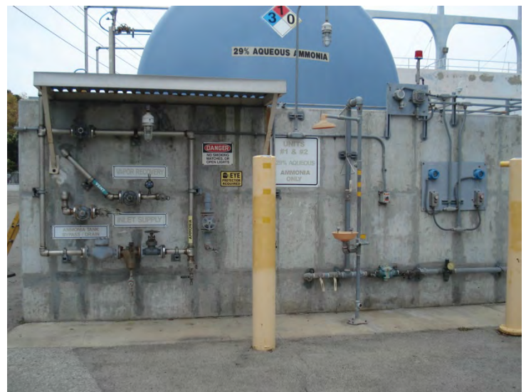
Photograph 5: 29% Aqueous ammonia tank for Units 1 and 2.
