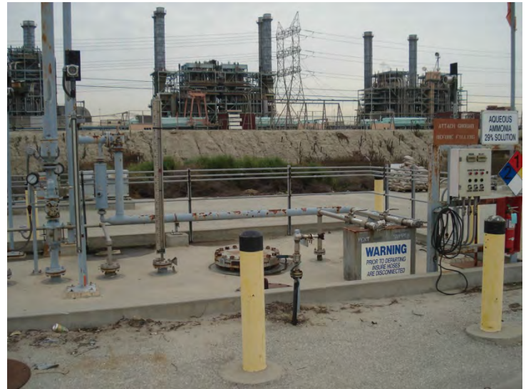
Photograph 16: Underground aqueous ammonia storage tank for Units 5 and 6.
