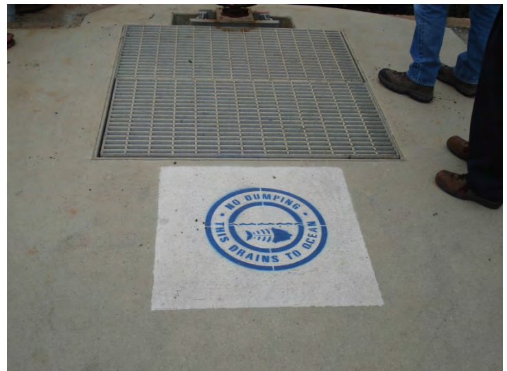
Photograph 6: Normal storm water runoff drain.
