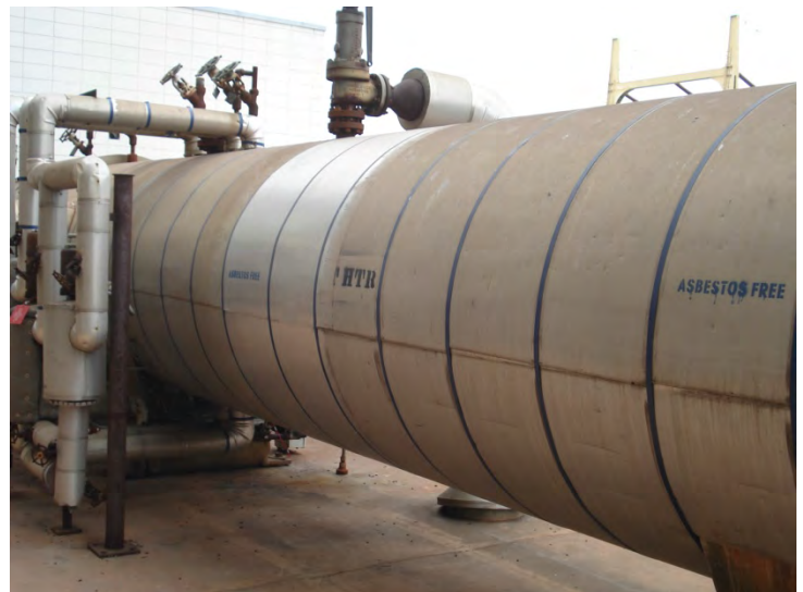
Photograph 24: Insulated equipment with blue straps and "asbestos free" notification.
