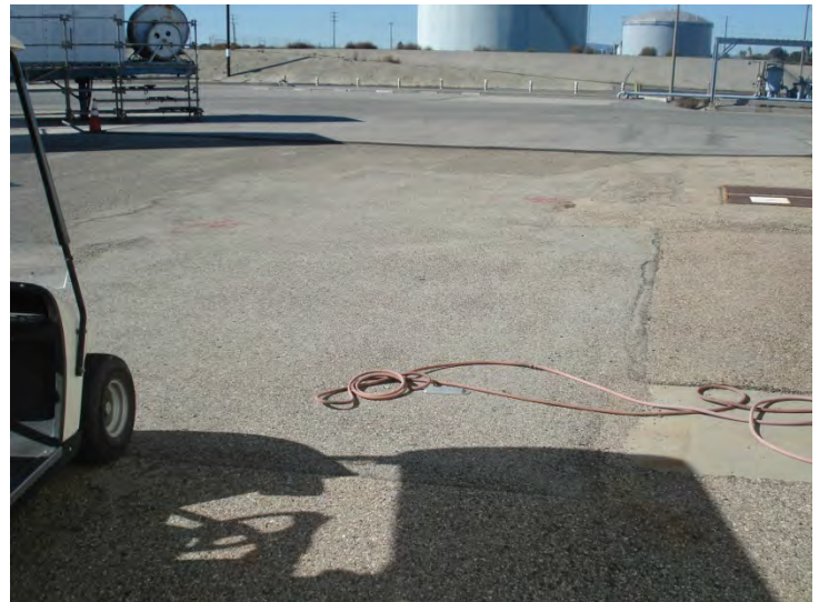
Photograph 33: Former UST area to the south of the electric shop.
