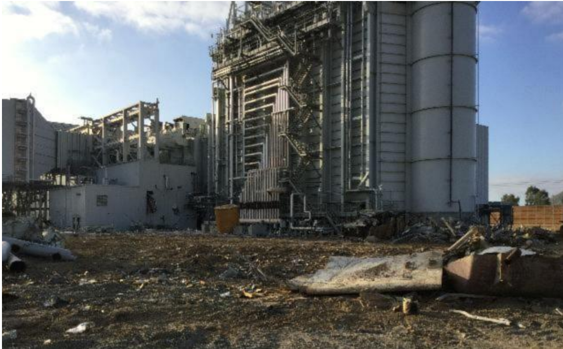
2020/05/11 06:55:20 Debris being cleared from in front of Unit 2.
