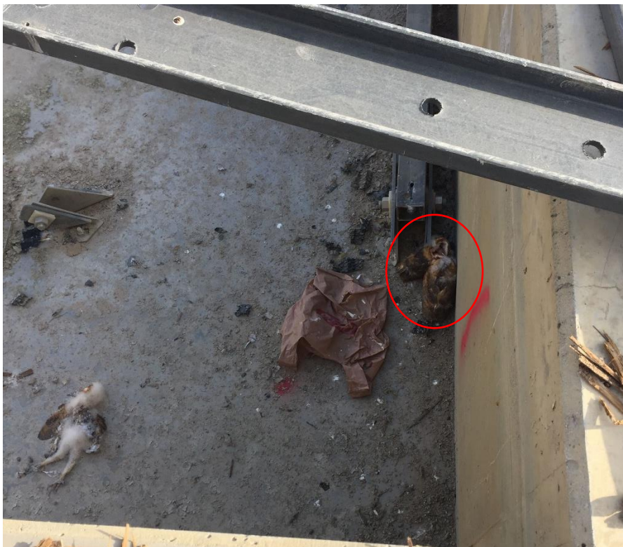
One dead owl chick (left) and two live chicks (circled) in cooling tower basin.
