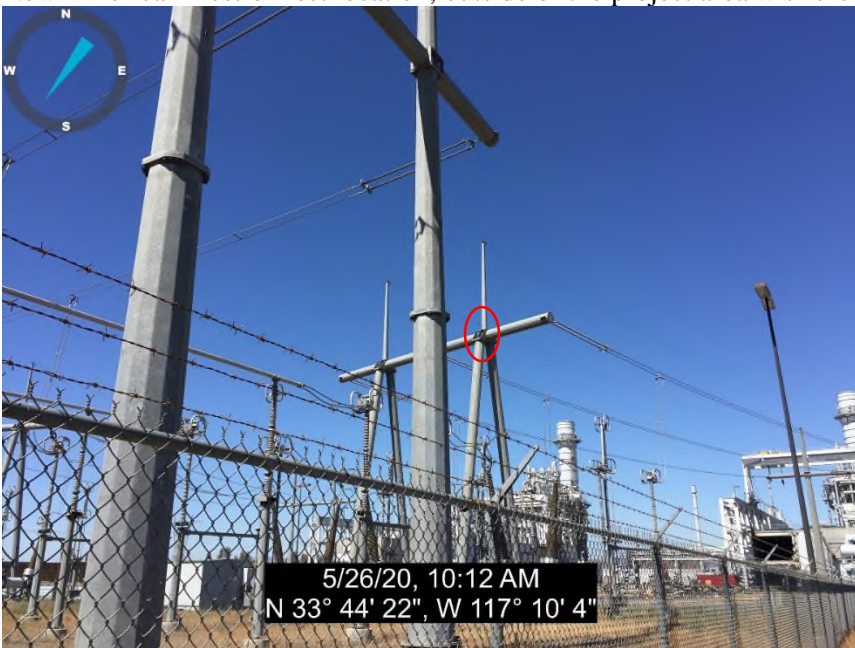
Location of stick nest observed (likely raven) within switch yard.
