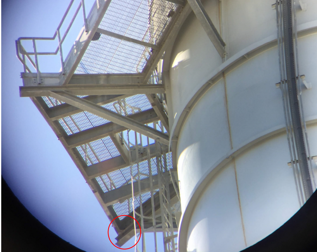
Location of kingbird nesting material removed from Unit 1 stack catwalk.
