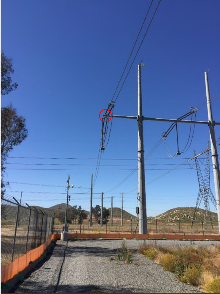
New American Kestrel nest location, outside of the project area with the arm of the transmission tower.
