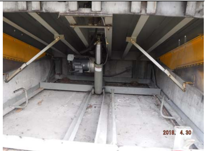
Photo 26: View below the hydraulic lift.
