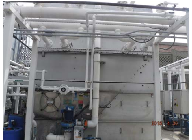
Photo 22: View of a chiller.
