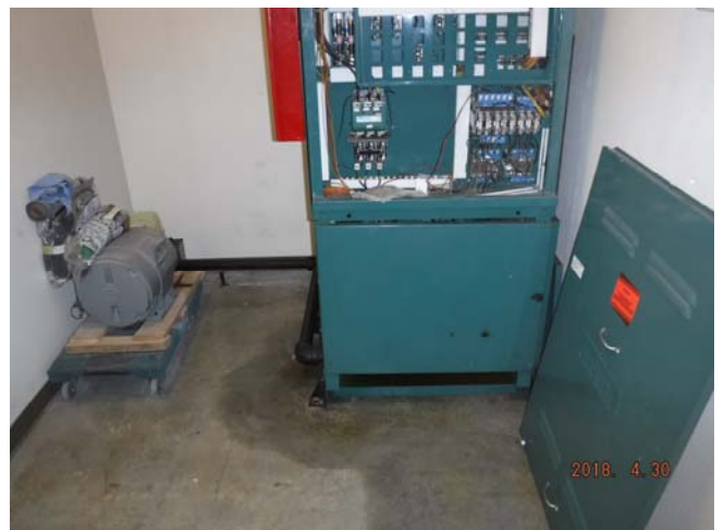
Photo 24: Staining next to the hydraulic elevator equipment.
