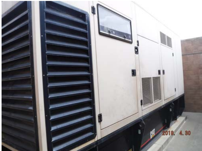
Photo 21: View of the 650-gallon diesel AST.
