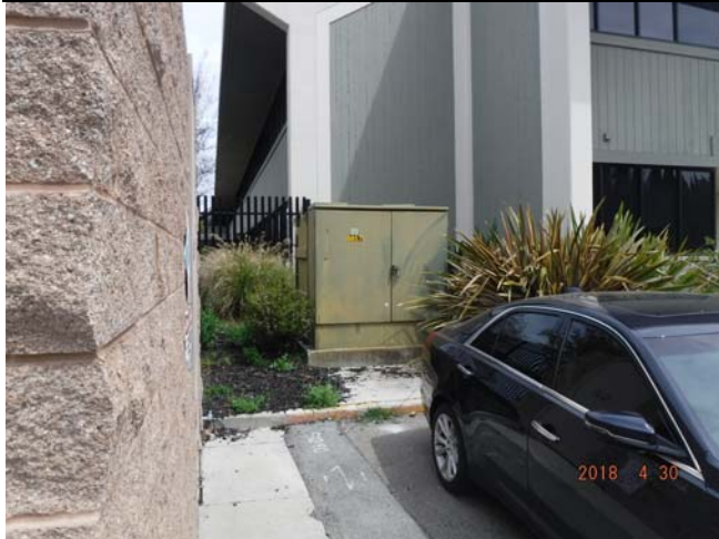
Photo 19: View of a pad-mounted transformer.
