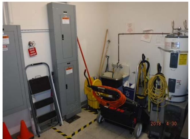
Photo 12: View of a janitorial closet.
