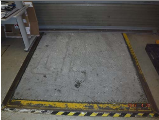
Photo 25: View of a hydraulic lift.
