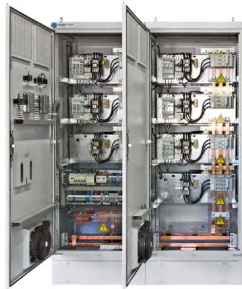
Figure 9: Facility-scale harmonic filter in housed in cabinets.
