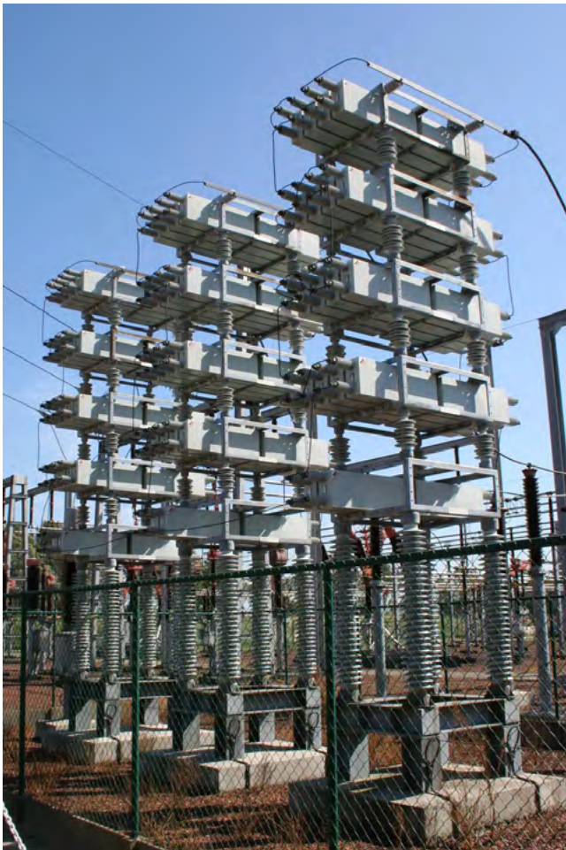
Figure 8: A 75 MVAR (million volt-amp reactive) capacitor bank installed at a utility substation.
