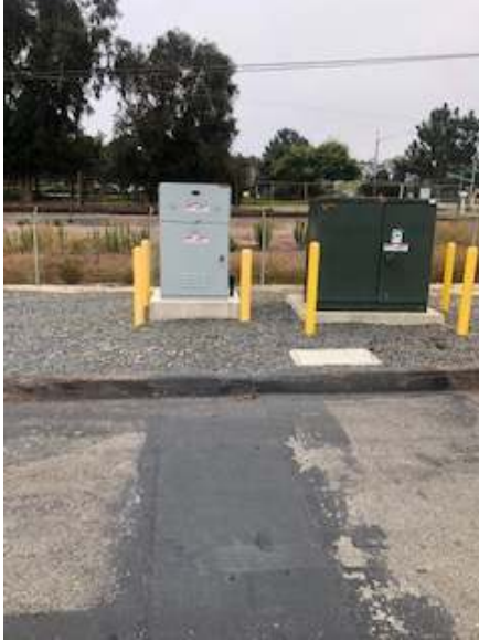
South Ingress Curb, Gravel, Driveway, Bollards and Electrical Units facing East
