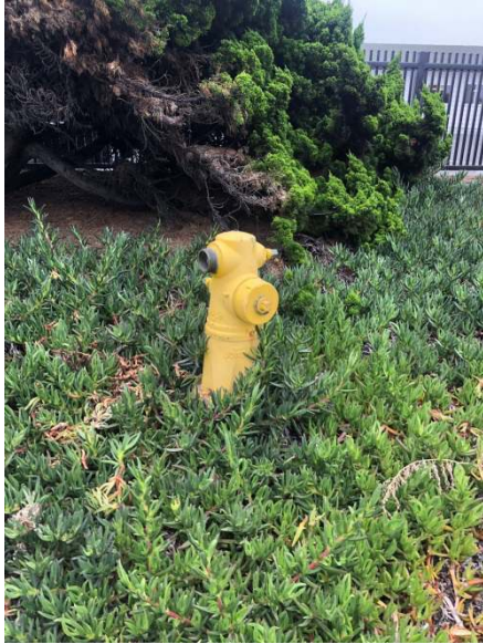
Fire Hydrant and Plants at Northeast Ingress
