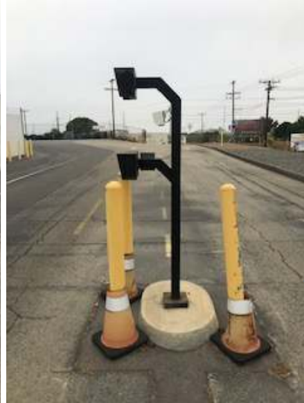
South Egress Card Reader facing North
