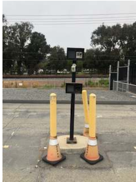
South Egress Card Reader facing East
