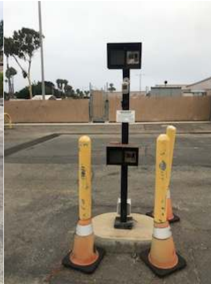
South Ingress Card Reader facing West
